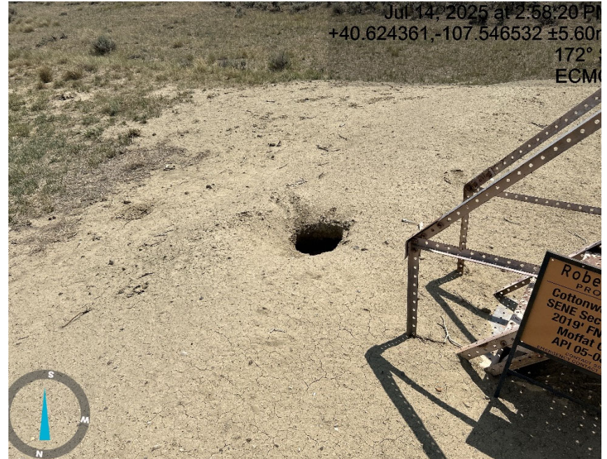
Holes in containment
