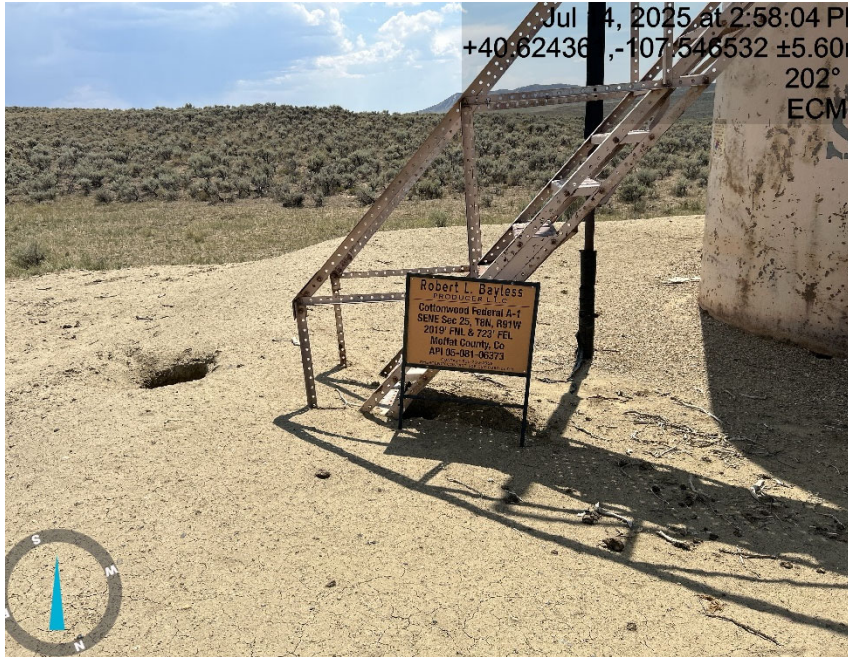
Tank battery signage
