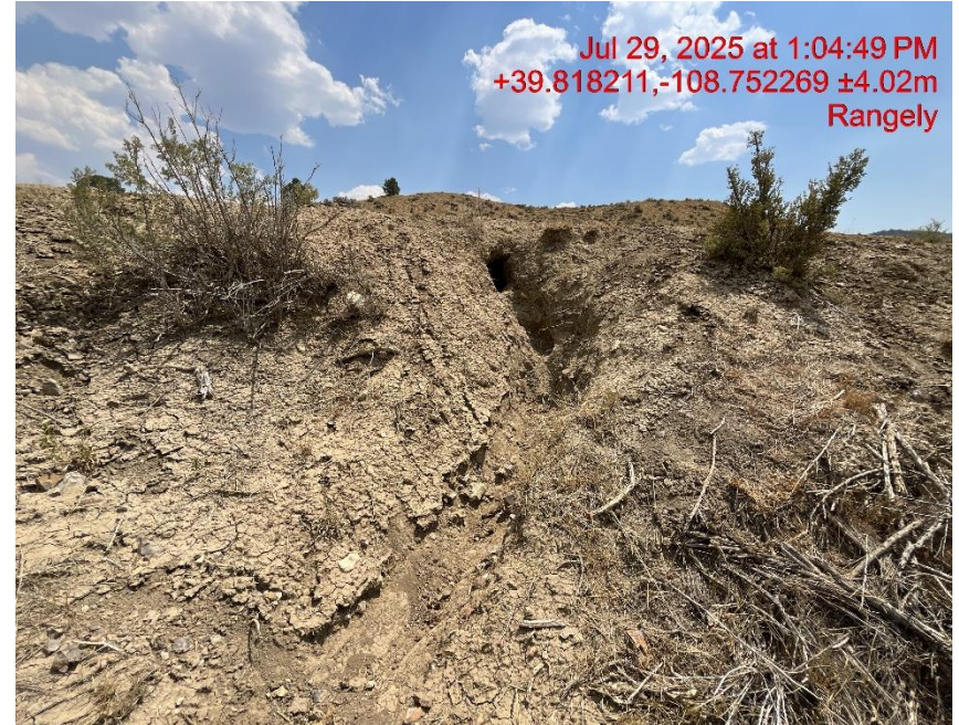
Photo # 0982 Tunnel erosion/Berm needs maintenance
