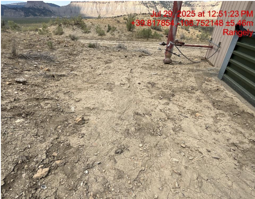
Photo # 0968 Failure to minimize erosion & transport of sediment
