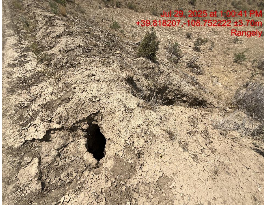
Photo # 0977 Tunnel erosion/Berm needs maintenance
