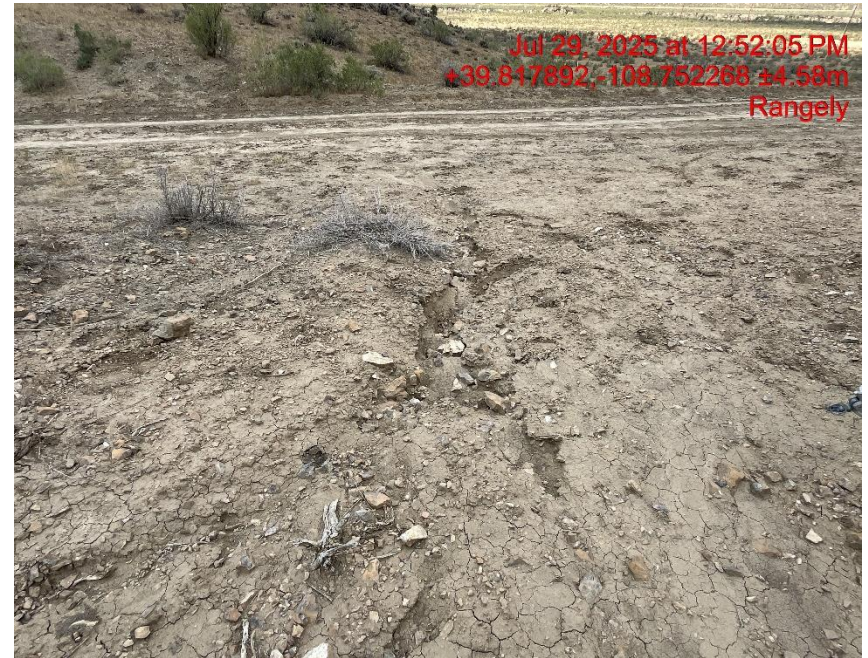
Photo # 0970 Failure to minimize erosion & transport of sediment
