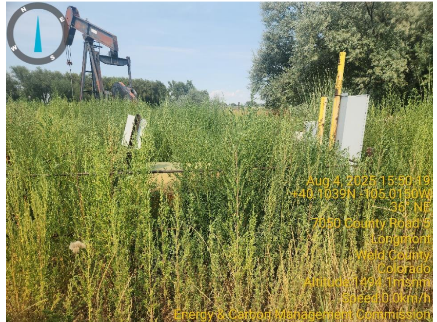
Photo 4 Ancillary equipment over run with tall vegetation.
