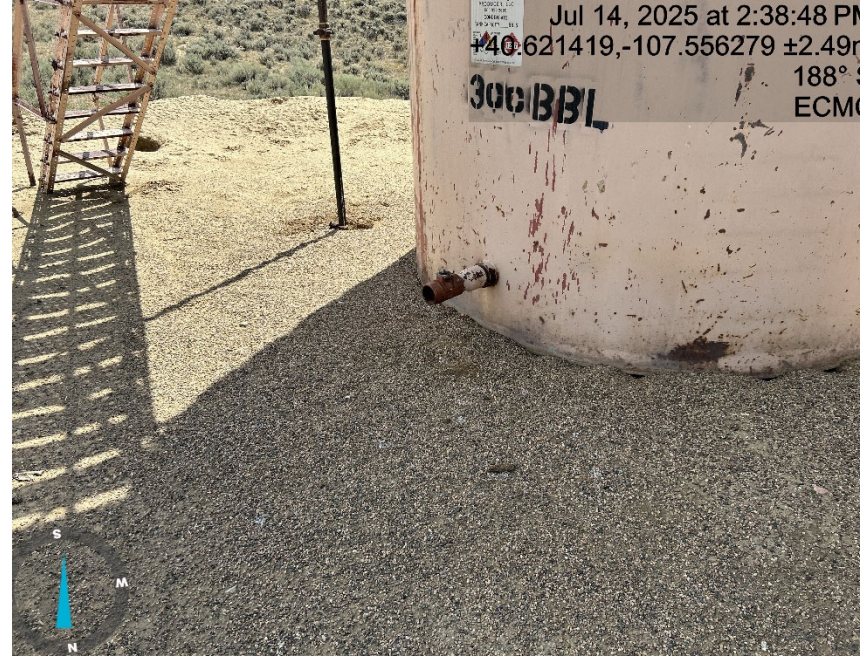
Open load line
