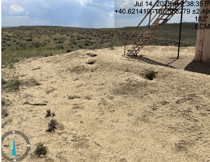
Holes in containment
