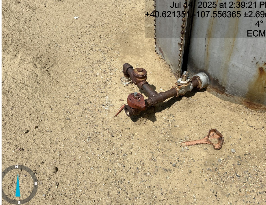
Open load line
