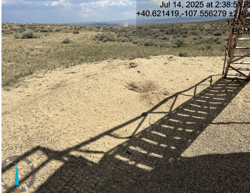
Holes in containment
