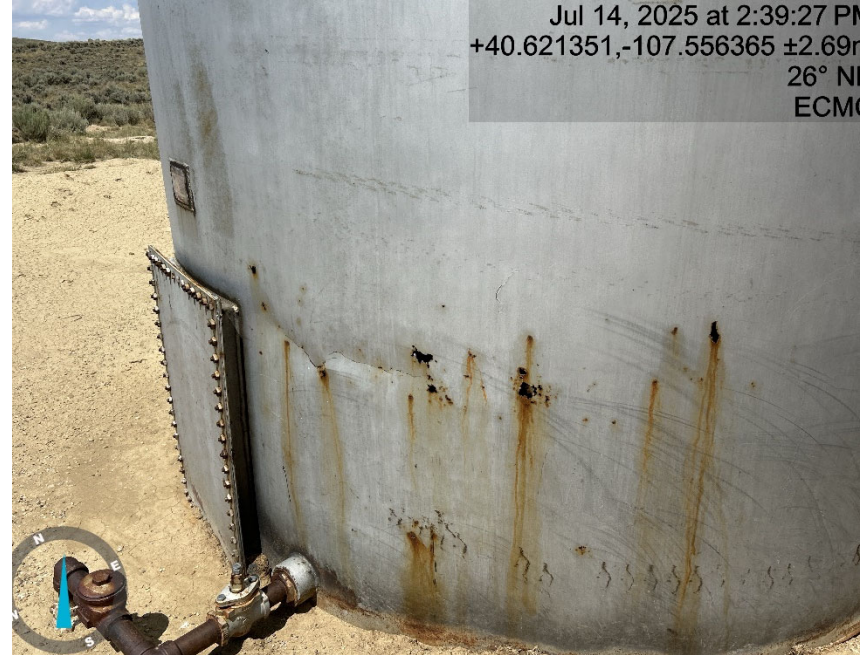
Multiple holes in tank
