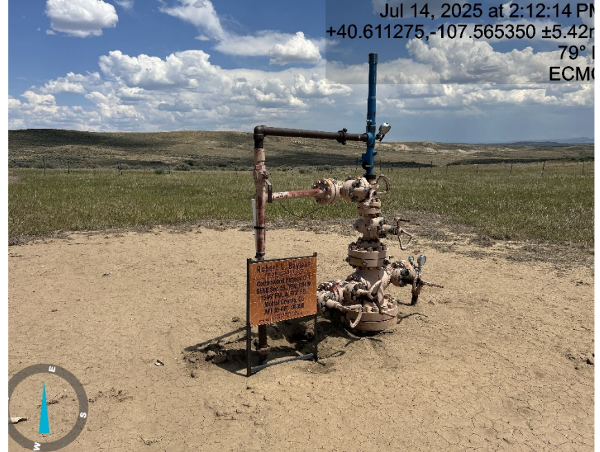
Location/ well signage is becoming illegible.
