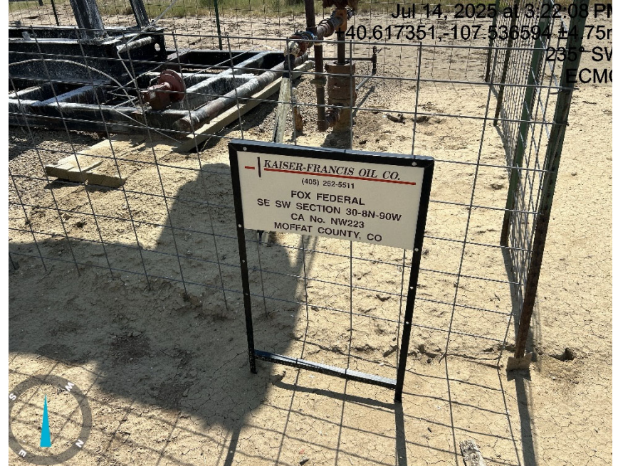
Well signage lacks information
