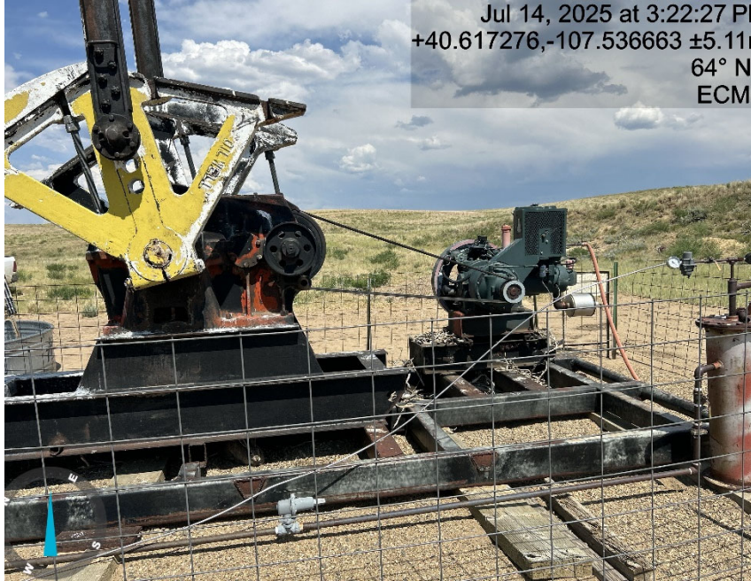
Belt guard missing
