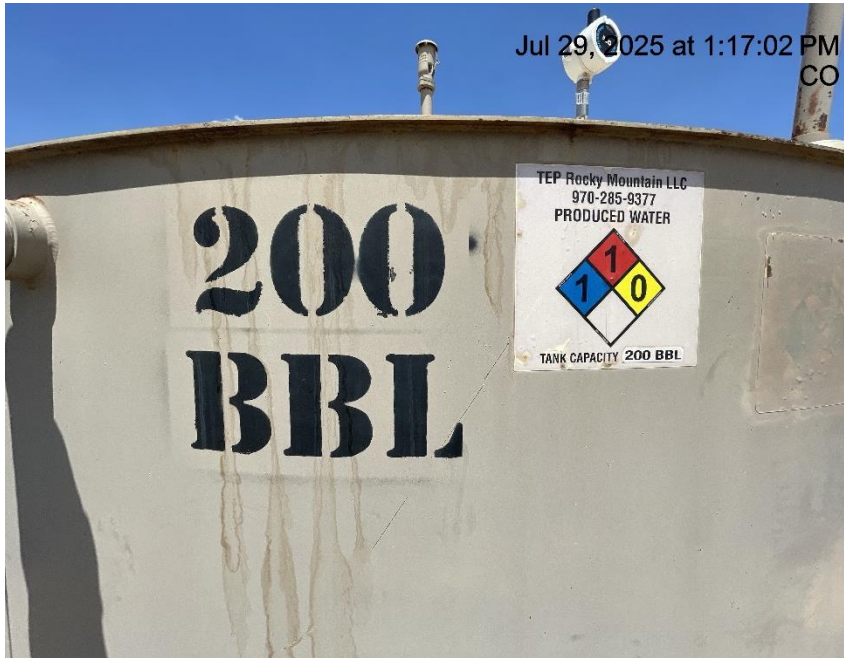
Photo # 5695 Tank capacity incorrect
