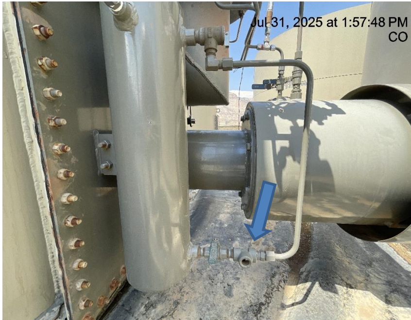
Photo # 6403 PRV vent line on tank burner does not comply with CECMC pressure safety device rules & general safety rules
