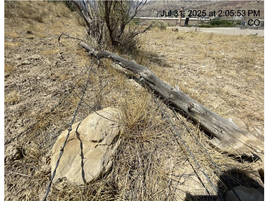
Photo # 6398 Barbed wire fence needs maintenance/wildlife hazard
