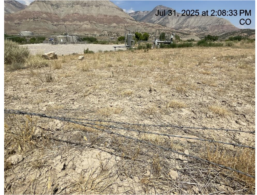
Photo # 6400 Barbed wire fence needs maintenance/wildlife hazard
