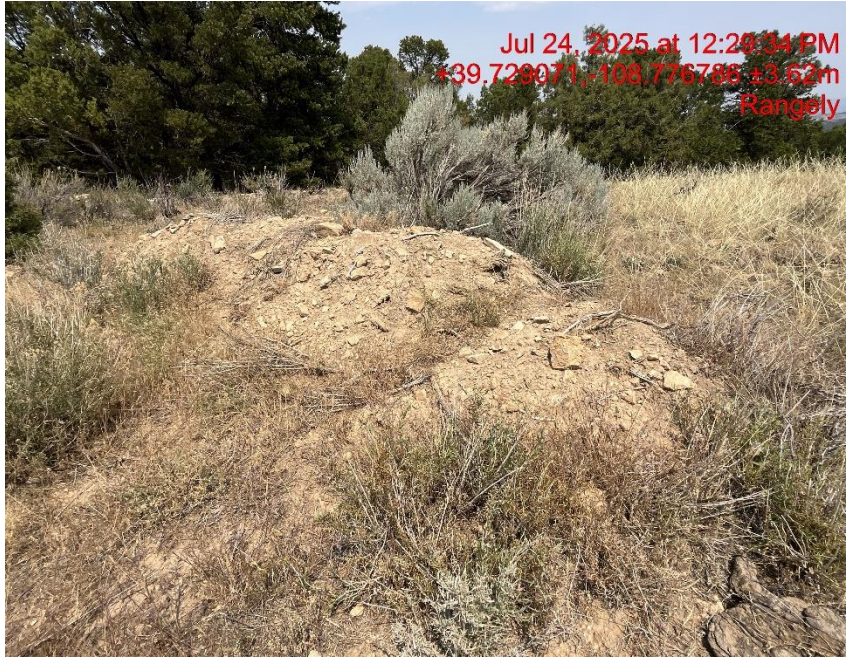
Photo # 0867 Stockpiled soils with no BMP's
