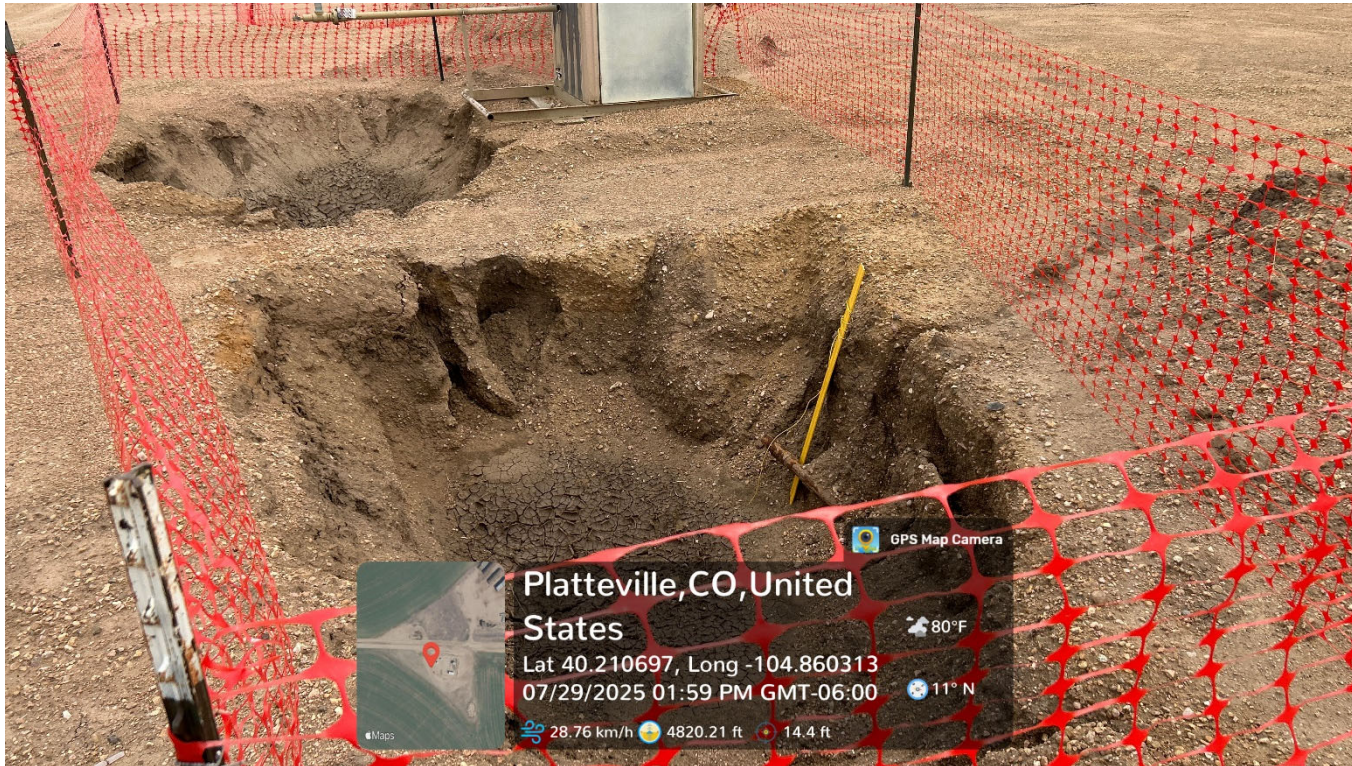
Photo 3 – Open excavation with abandoned pipe
