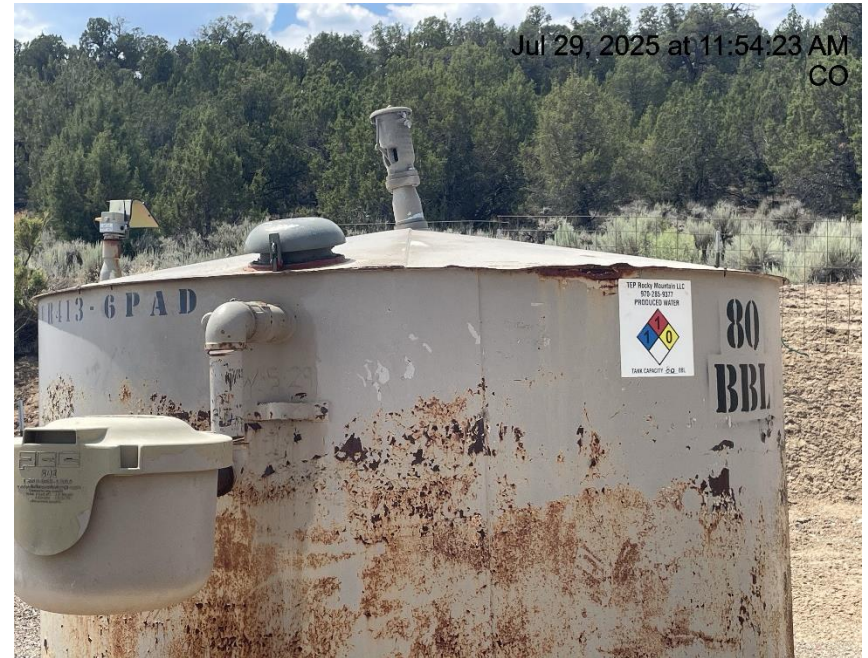
Photo # 5488 Production tank showing signs of corrosion
