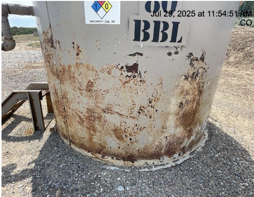
Photo # 5487 Production tank showing signs of corrosion
