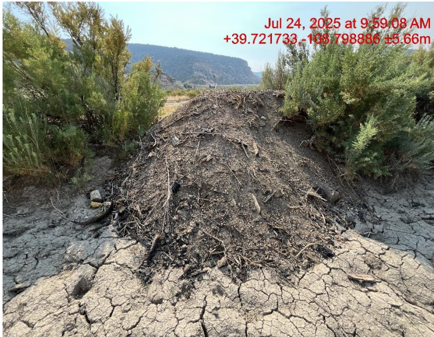
Photo # 0792 Stockpiled soils with no BMP's
