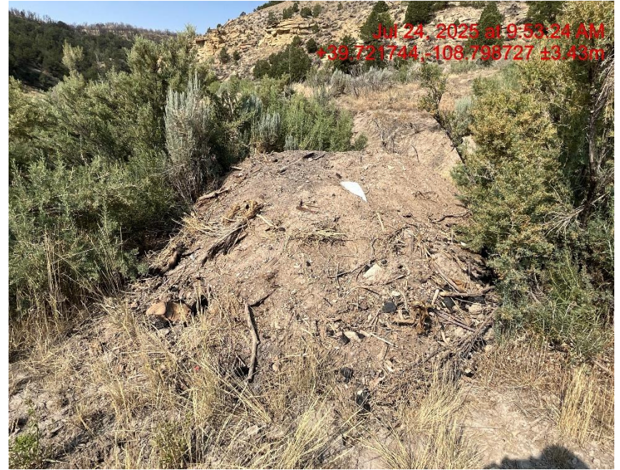
Photo # 0789 Stockpiled soils with no BMP's
