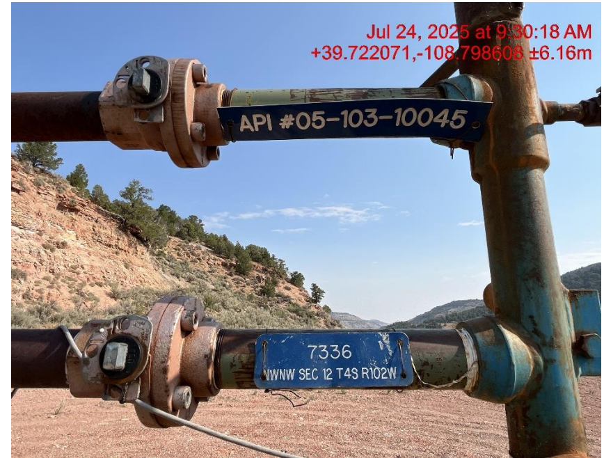
Photo # 0773 Wellhead sign lacks required information/not in compliance with CECMC rules
