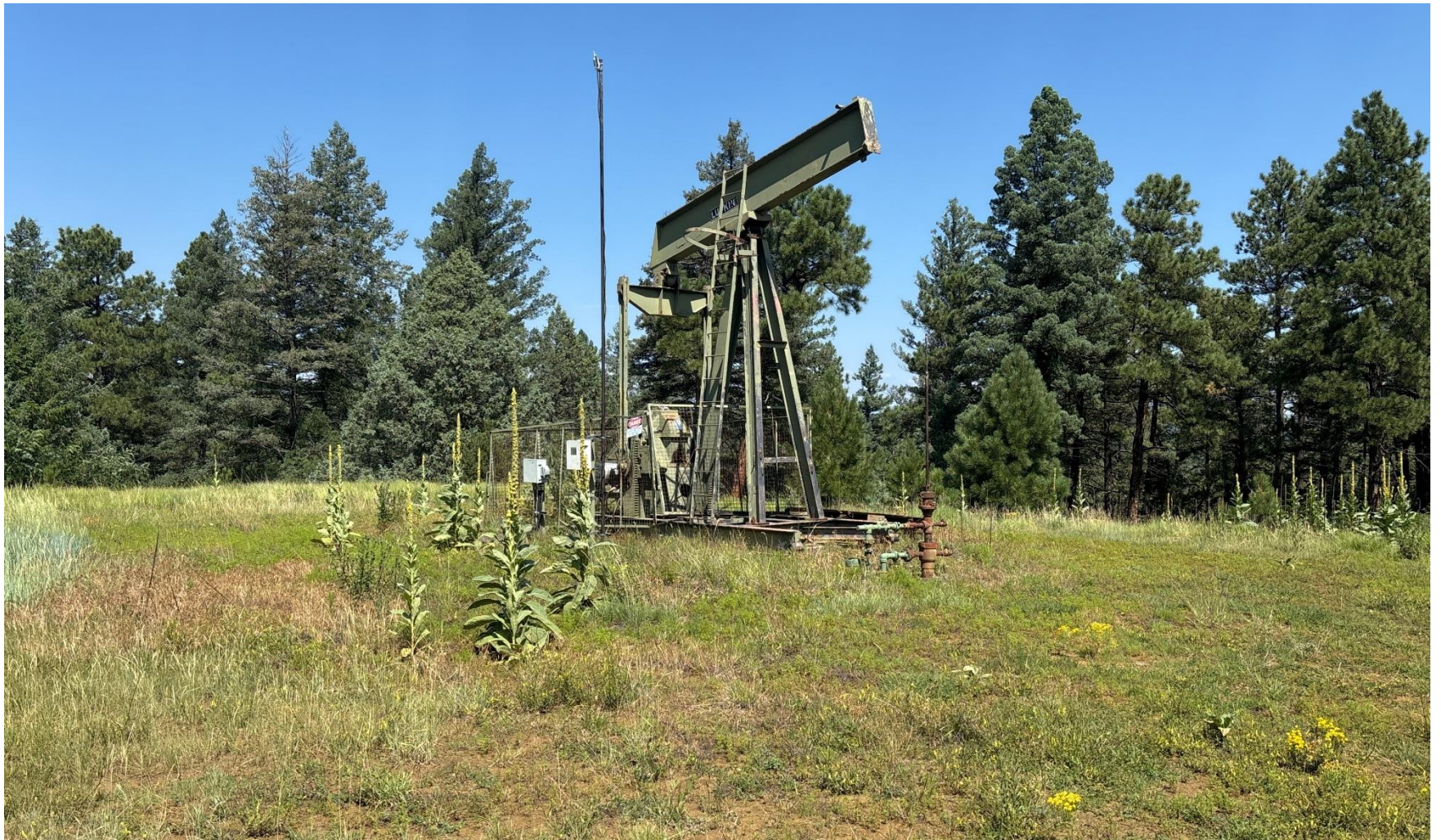
PHOTO 3: WELLHEAD AND EQUIPMENT/ THERE MUST BE A 20' RADIOUS CLEAR OF WEEDS AROUND WELLHEAD AND EQUIPMENT. MAINTAIN WEEDS PER RULE 606.
