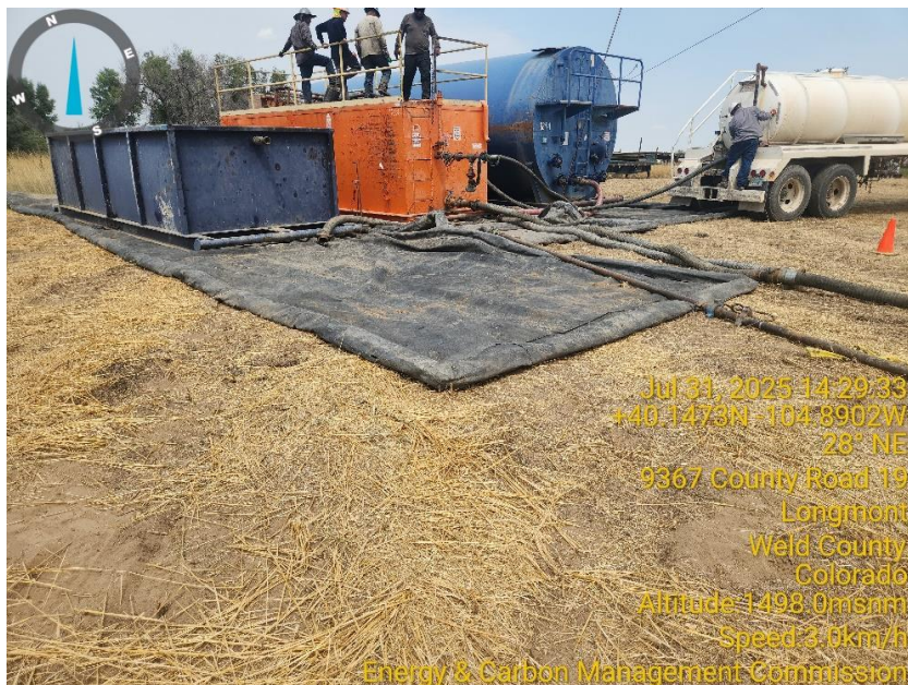
Photo 5 Circulation tank, fresh water tank.
