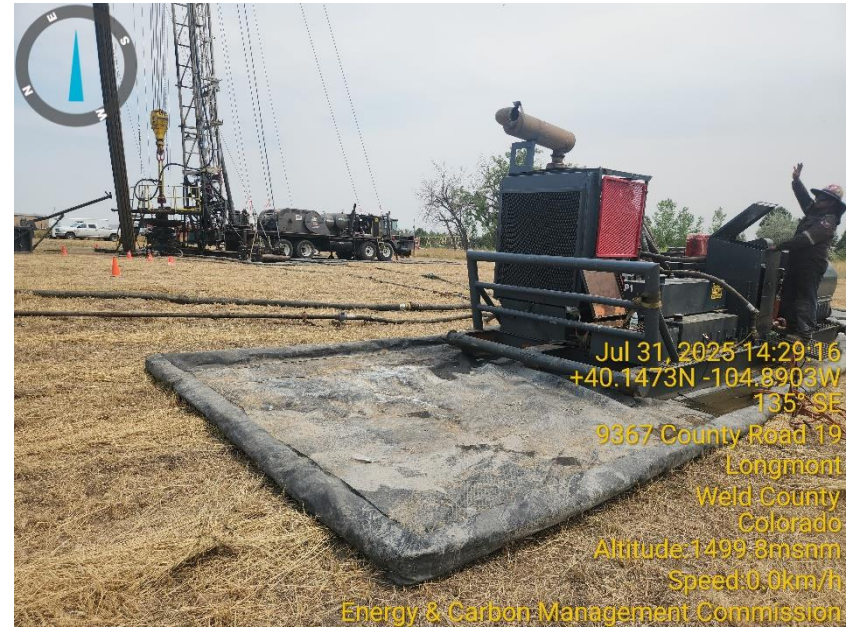
Photo 4 WO rig pump.
