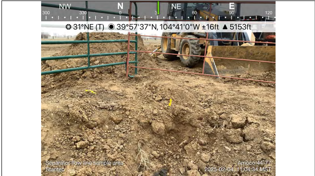
Photo #3 View of the flowline @ separator sample location
