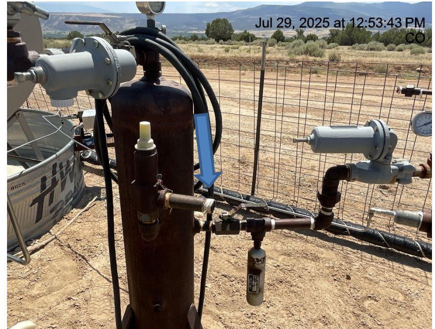
Photo # 5657 PRV vent line on domestic tap does not comply with CECMC pressure safety device rules & general safety rules
