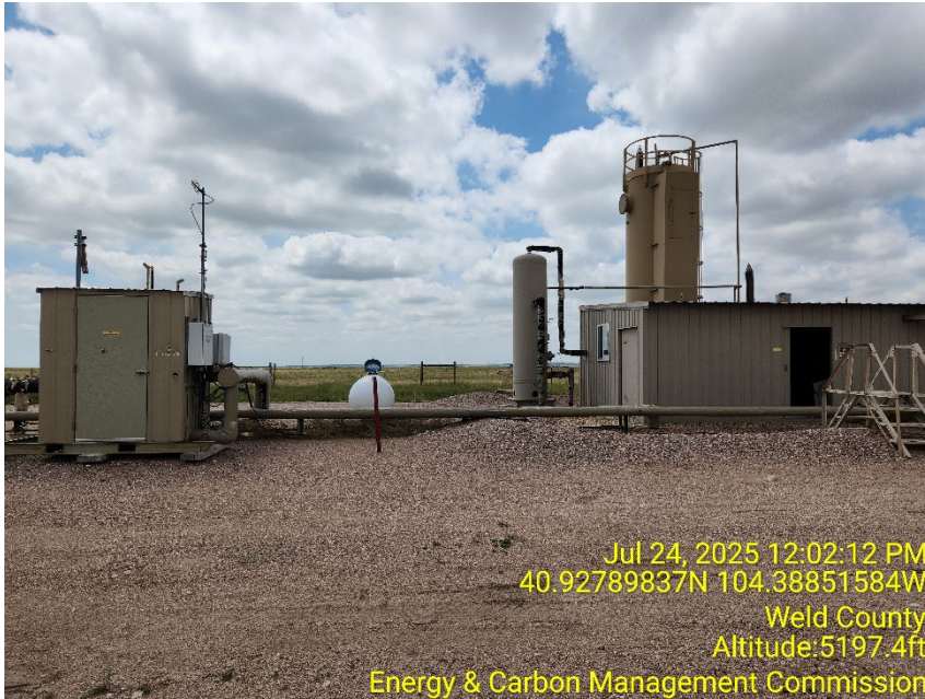
Photo 5 – Gas Meter, Heater Treater
