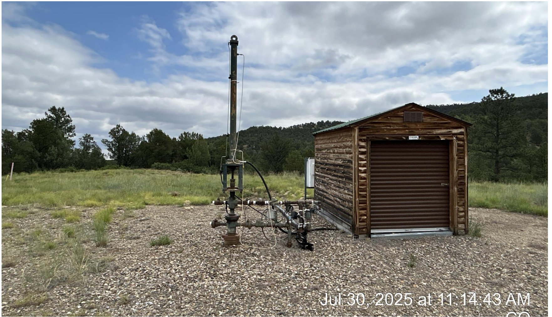
PHOTO 3: WELLHEAD AND EQUIPMENT
