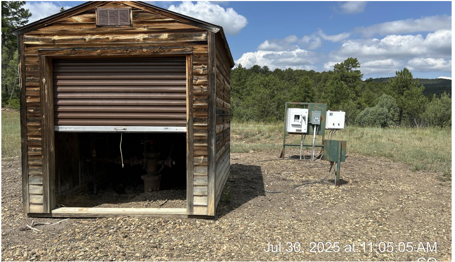
PHOTO 3: WELLHEAD AND EQUIPMENT
