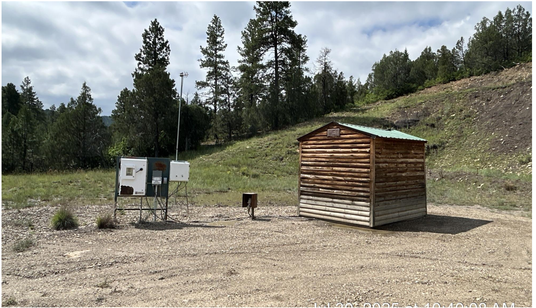
PHOTO 3: WELLHEAD AND EQUIPMENT
