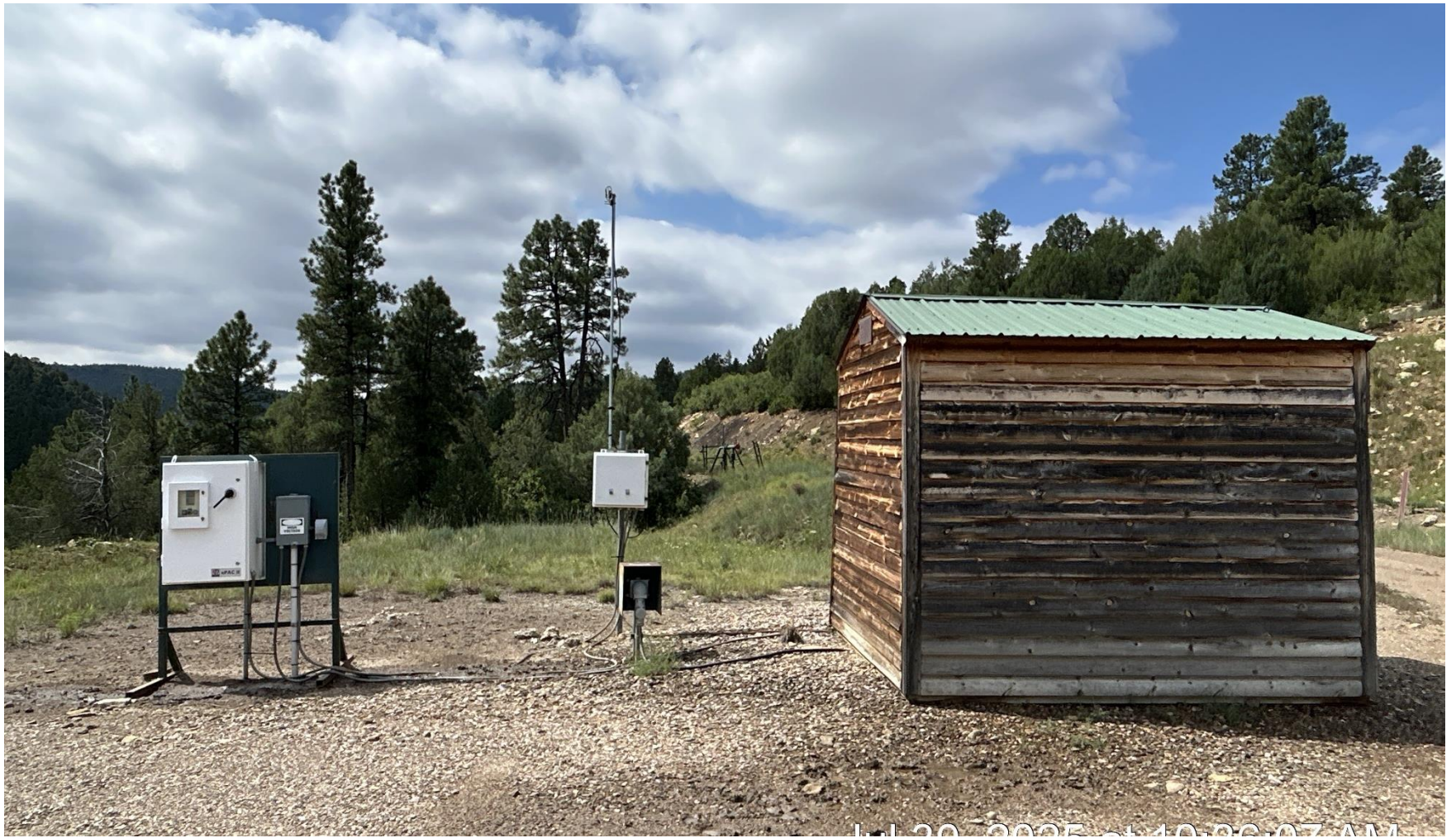
PHOTO 3: WELLHEAD AND EQUIPMENT
