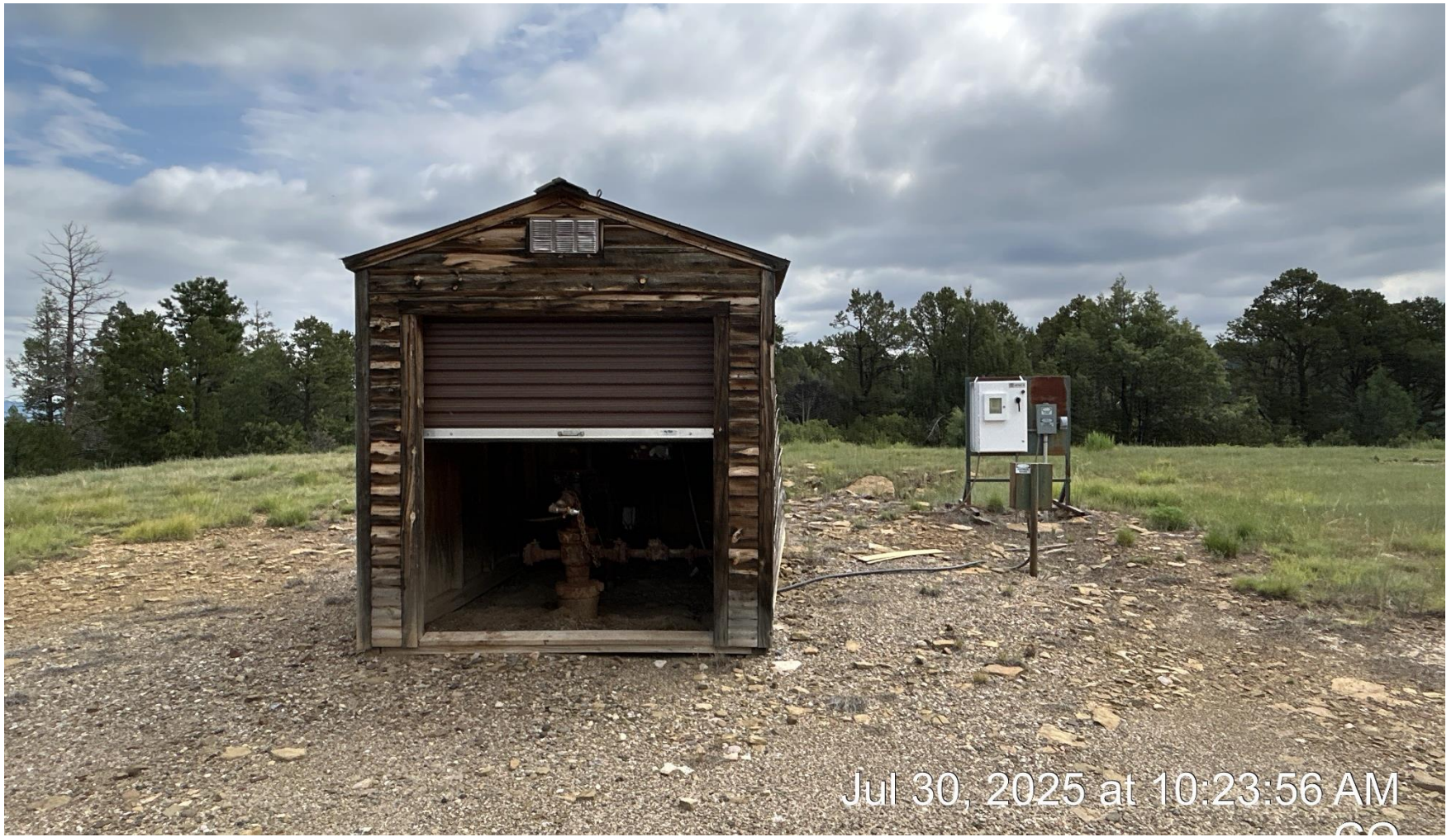
PHOTO 3: WELLHEAD AND EQUIPMENT
