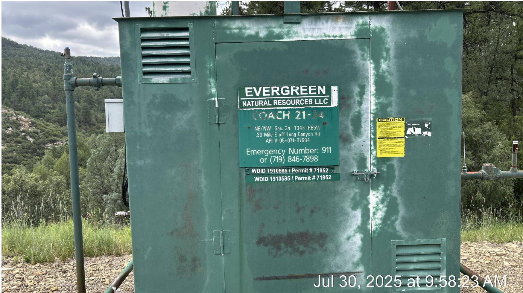
PHOTO 1: WELL SIGN NEEDS TO BE REOLACED
