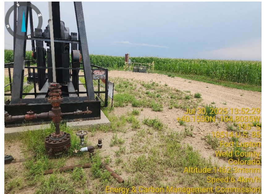
Photo 4 wellsite & ancillary equipment.
