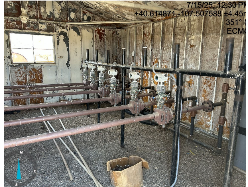
Lack of meter calibration cards
