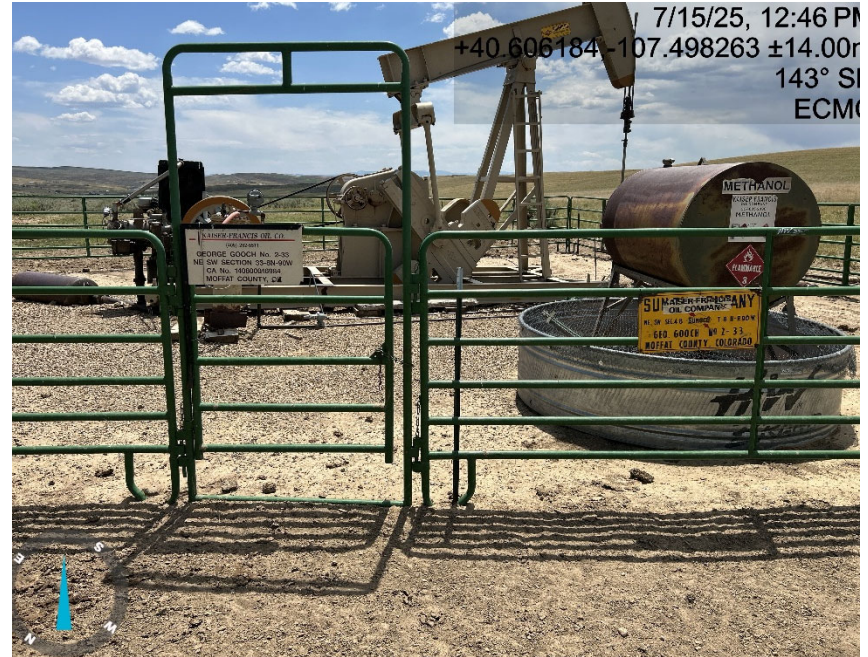
Well signage lacks information
