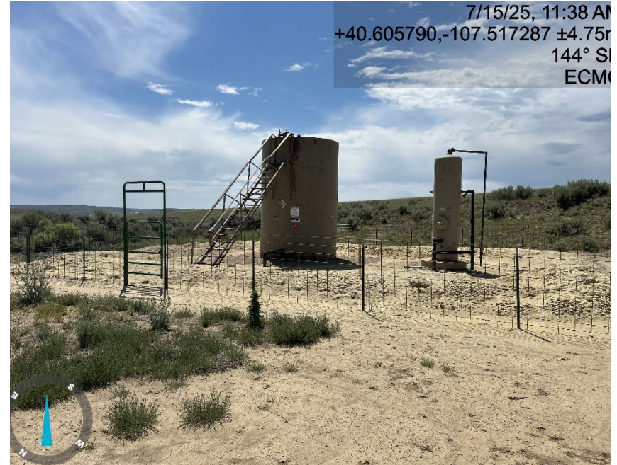
Tank battery signage is missing
