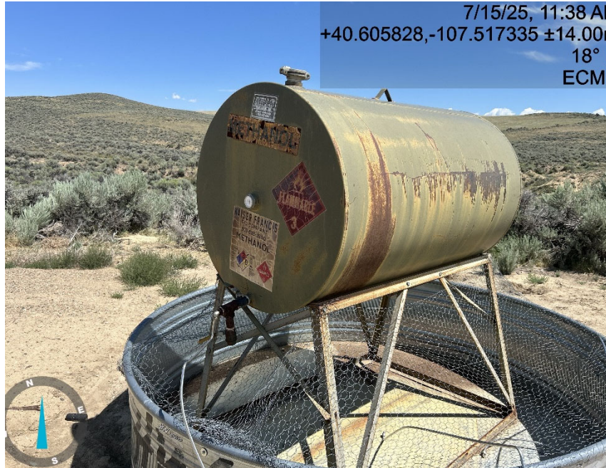
Chemical tank signage is fading
