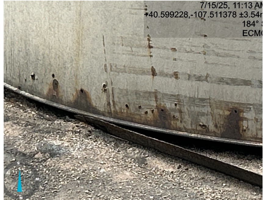
Multiple holes at base of tank
