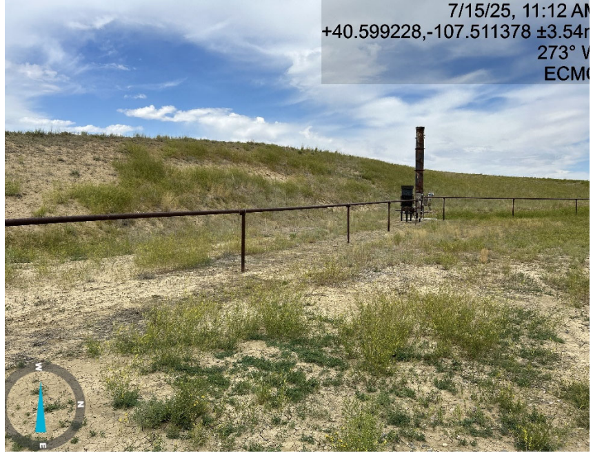
Location and ECD's are not running and not metered
