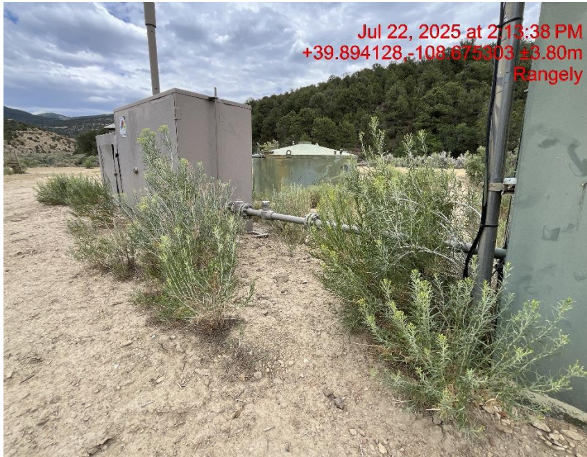
Photo # 0620 Weeds/undesirable plant species surrounding production equipment constitutes a fire hazard
