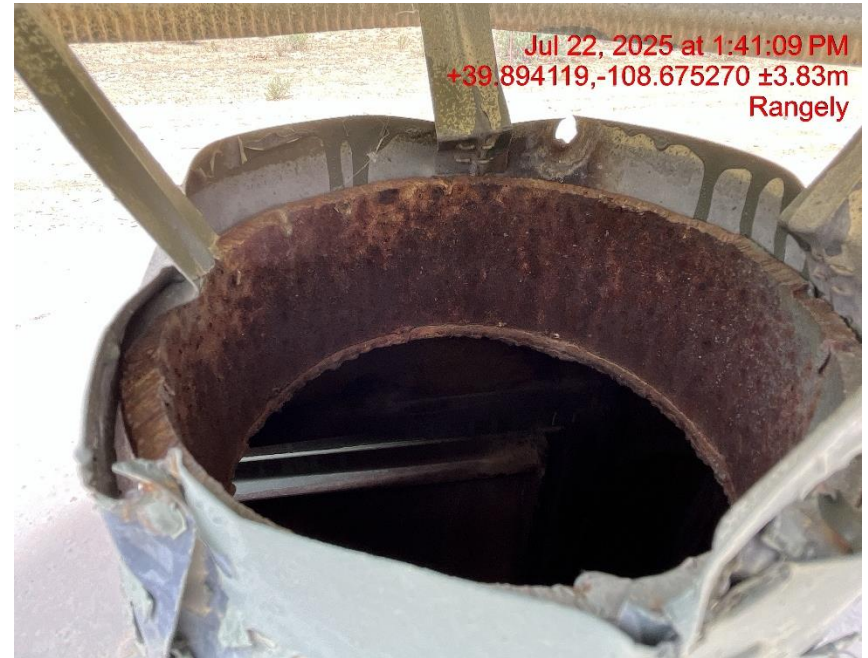
Photo # 0595 Wildlife hazard
