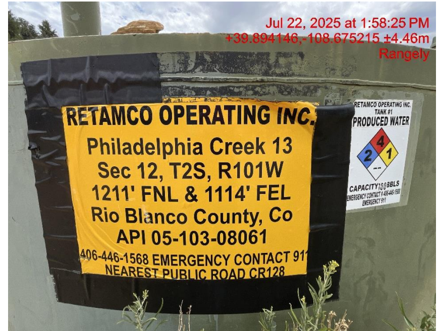
Photo # 0609 Battery sign lacks quarter/quarter section information/not in compliance with CECMC rule
