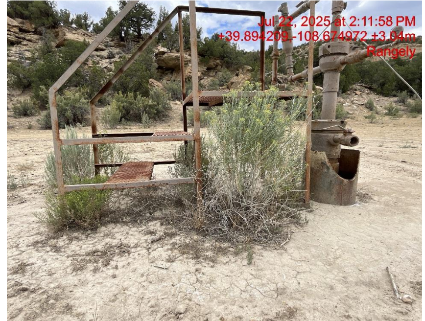
Photo # 0618 Weeds/undesirable plant species surrounding production equipment constitutes a fire hazard
