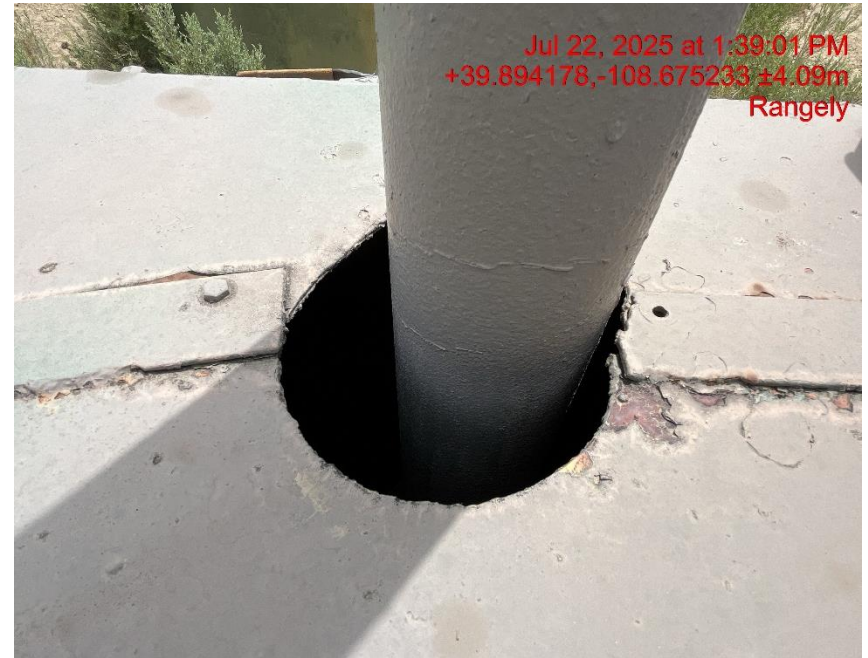
Photo # 0593 Wildlife hazard
