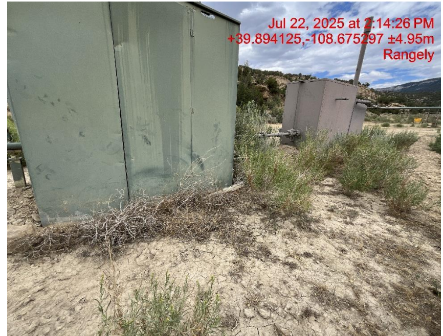
Photo # 0621 Weeds/undesirable plant species surrounding production equipment constitutes a fire hazard
