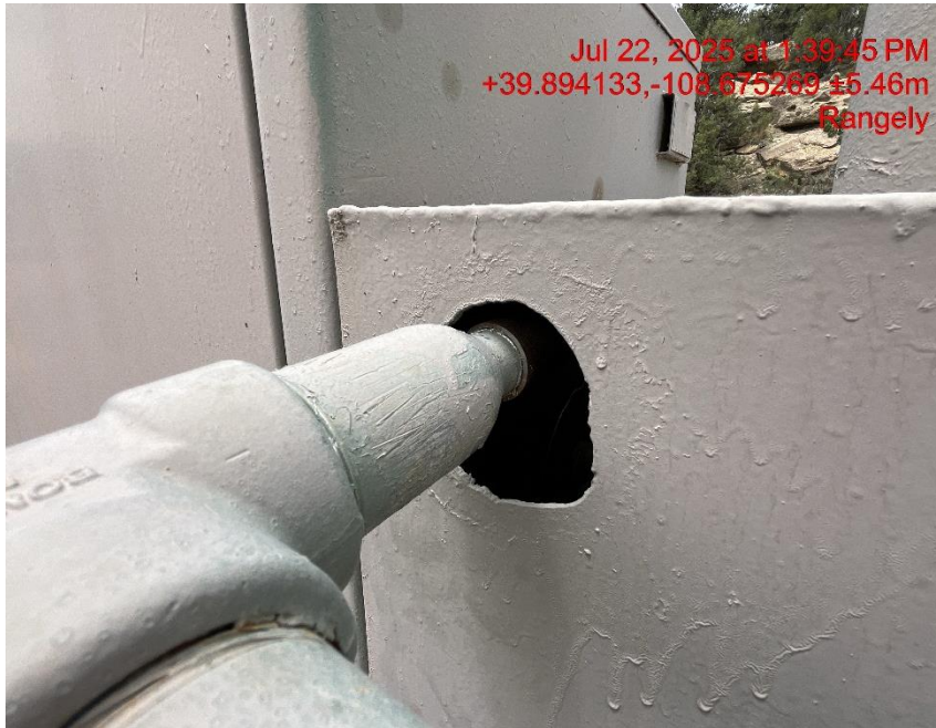
Photo # 0594 Wildlife hazard
