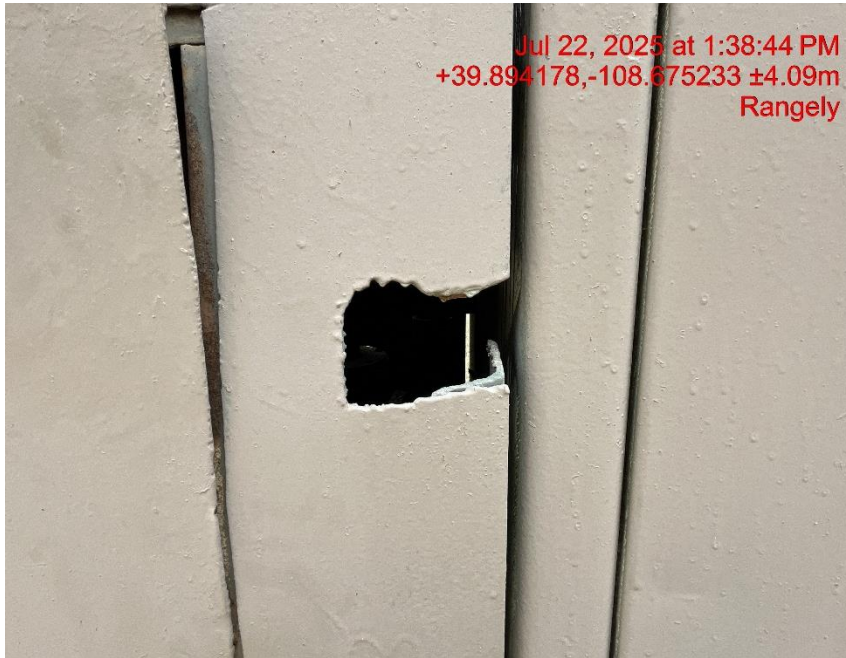
Photo # 0592 Wildlife hazard
