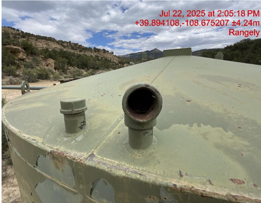
Photo # 0614 Open ended piping on tank/wildlife hazard/available for entry by wildlife
