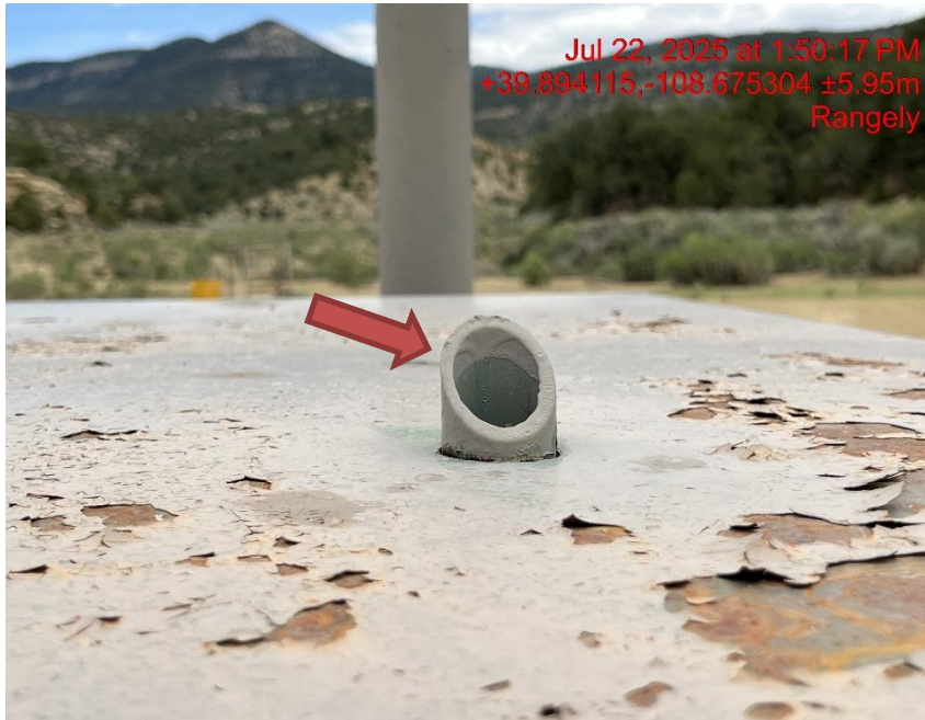
Photo # 0600 PRV vent line does not comply with CECMC pressure safety device rules
