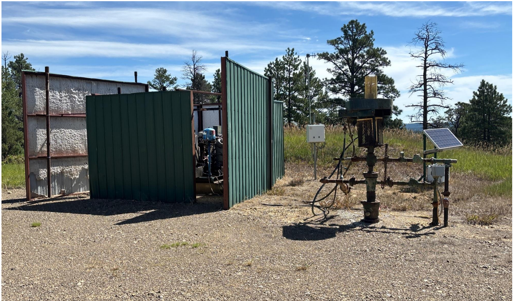
PHOTO 3: WELLHEAD AND EQUIPMENT.
