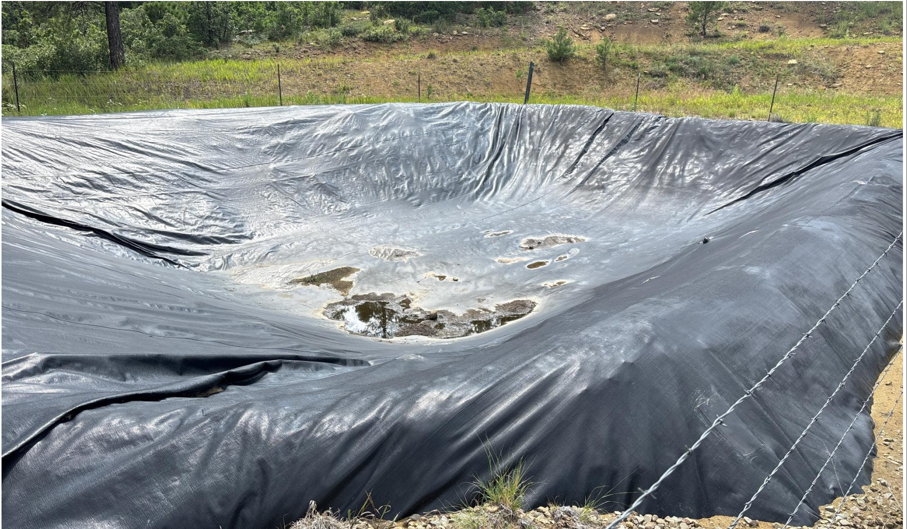
PHOTO 5: TR PRODUCED WATER PIT. THERE IS NO SYSTEM SET TO ALLOW WILDLIFE A WAY OUT OF LINED PIT. COMPY WITH RULE 909.b. Comply with general provisions of the oil and gas act for wildlife protection AND SB-181. (PROVIDE SOME WAY FOR WILDLIFE TO EXIT PIT).
