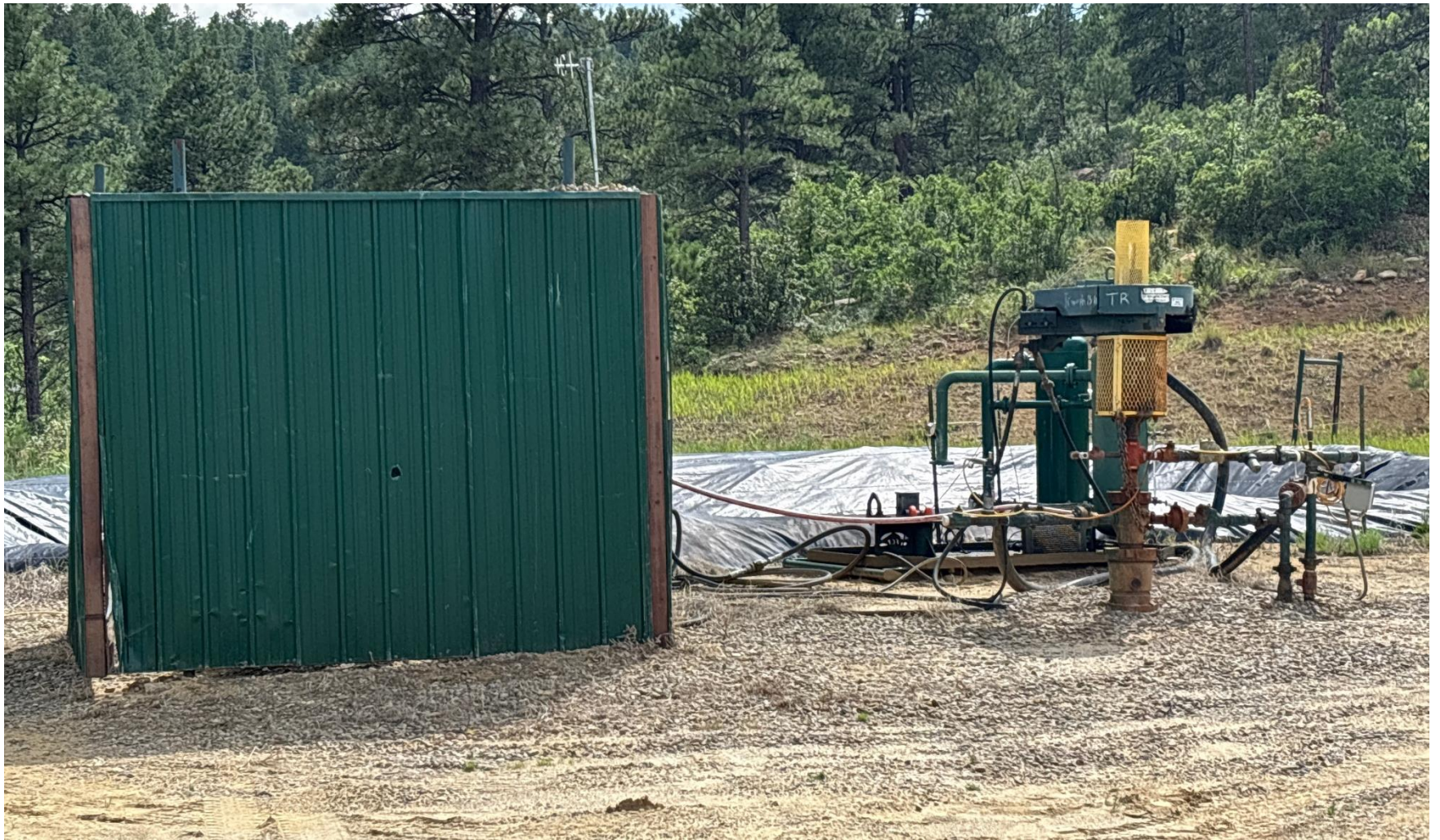
PHOTO 3: WELLHEAD AND EQUIPMENT.
