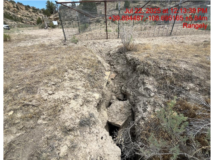
Photo # 0553 Failure to minimize erosion & transport of sediment off location/insufficient BMP's
