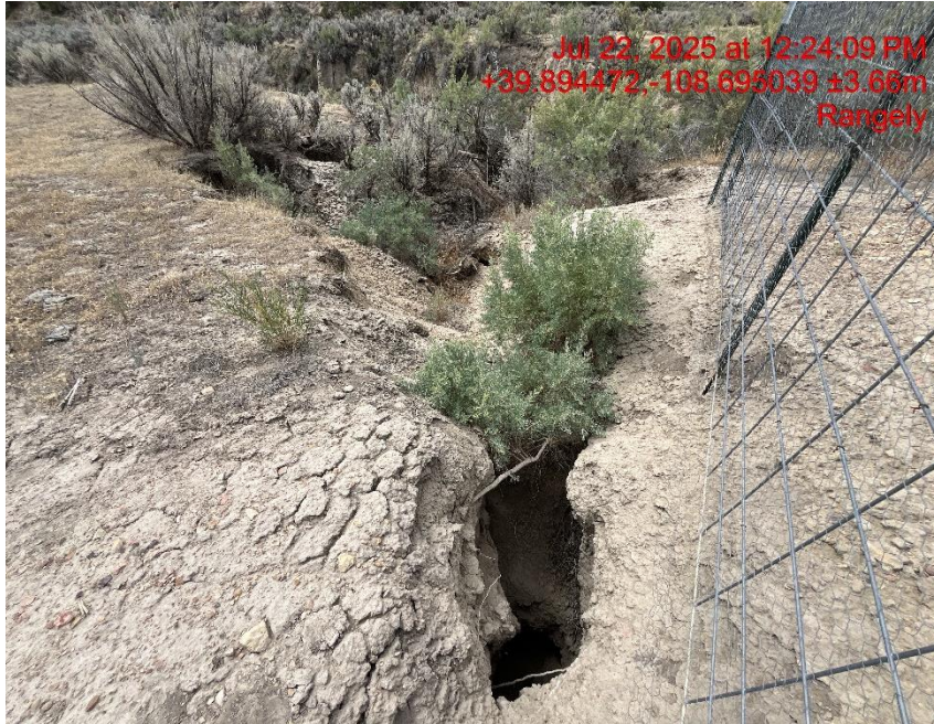
Photo # 0559 Failure to minimize erosion & transport of sediment off location/insufficient BMP's
