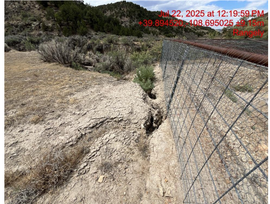
Photo # 0557 Failure to minimize erosion & transport of sediment off location/insufficient BMP's
