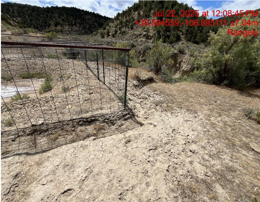
Photo # 0549 Failure to minimize erosion & transport of sediment off location/insufficient BMP's
