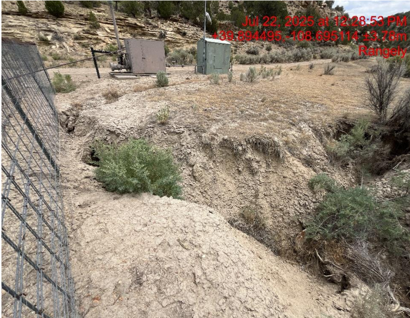
Photo # 0564 Failure to minimize erosion & transport of sediment off location/insufficient BMP's
