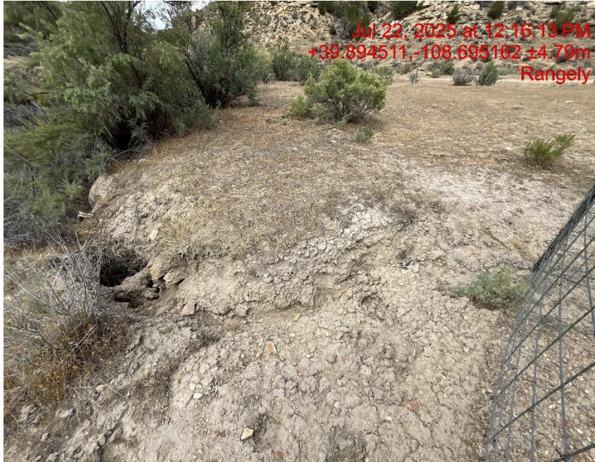
Photo # 0555 Failure to minimize erosion & transport of sediment off location/insufficient BMP's
