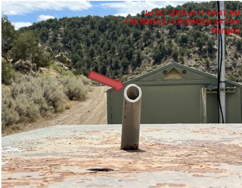
Photo # 0536 PRV vent line does not comply with CECMC pressure safety device rules
