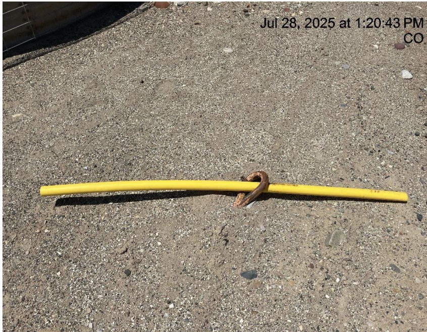
Photo # 5241 Improperly marked deadman
