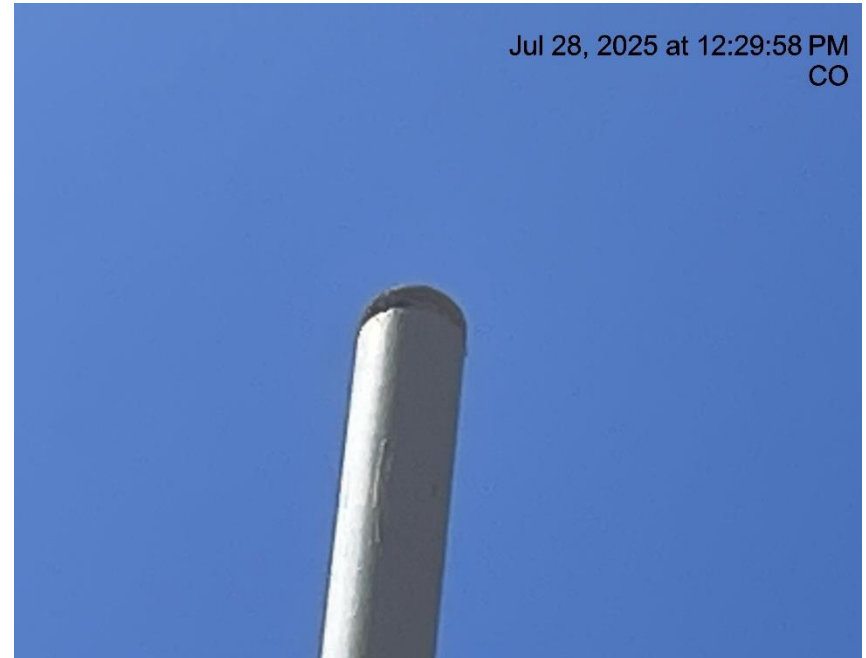
Photo # 5169 Open ended piping on dehy/wildlife hazard/available for entry by wildlife
