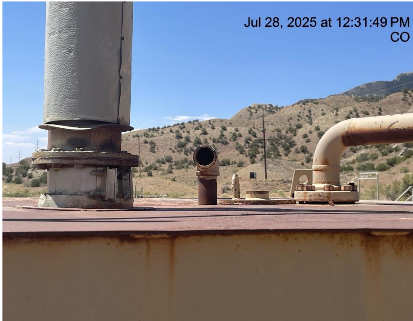
Photo # 5170 Open ended piping on dehy/wildlife hazard/available for entry by wildlife
