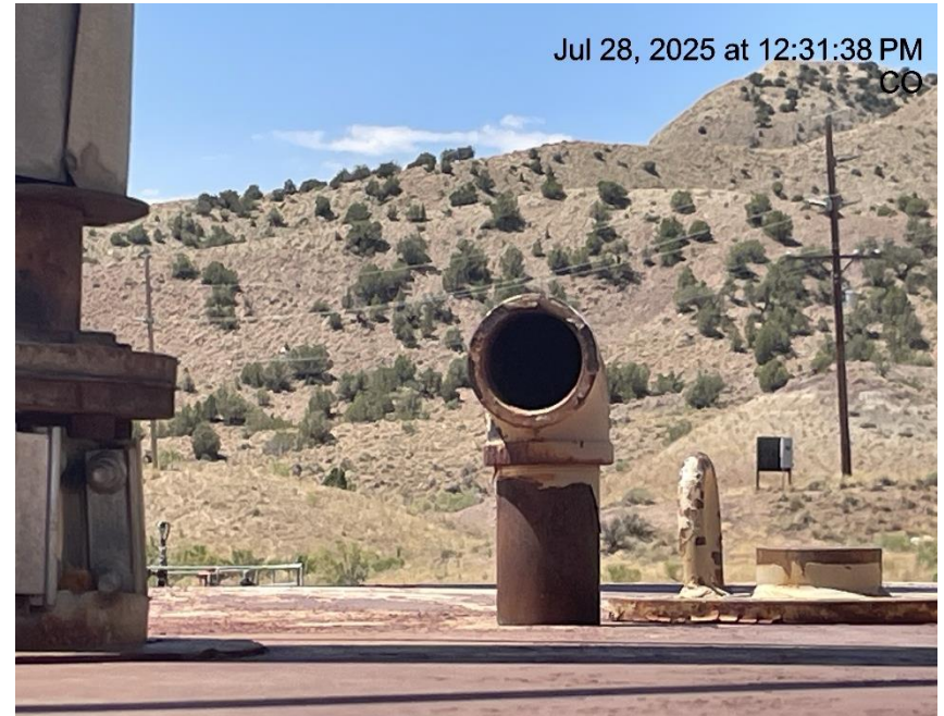
Photo # 5171 Open ended piping on dehy/wildlife hazard/available for entry by wildlife
