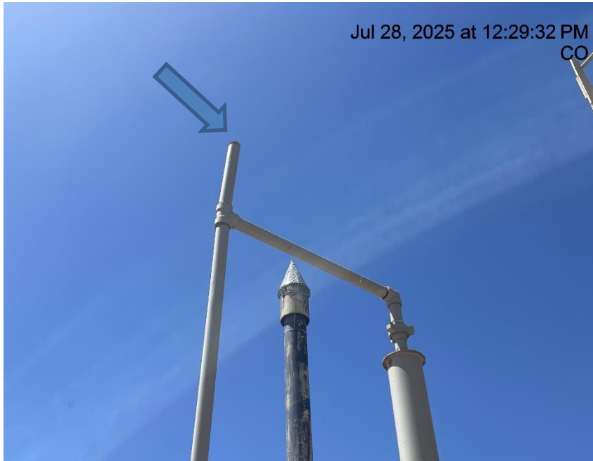
Photo # 5168 Open ended piping on dehy/wildlife hazard/available for entry by wildlife
