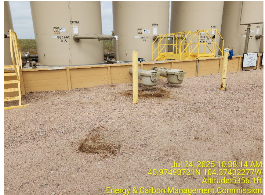
Photo 4 – Stained Soil at South Loadline Buckets
