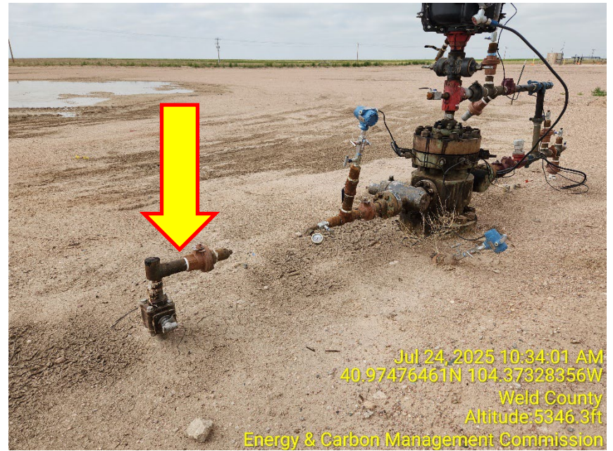
Photo 8 – Unused Riser – 25-2501H
