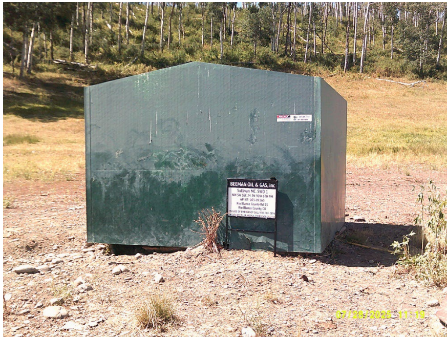
Injection wellhead inside housing
