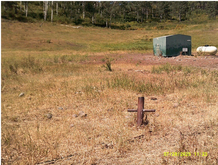
Unmarked guy line anchor
