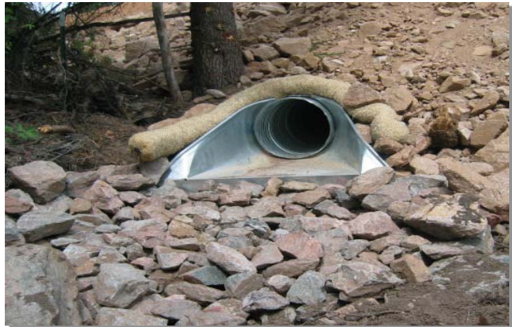
Photograph TOP-1. Riprap outlet protection.
