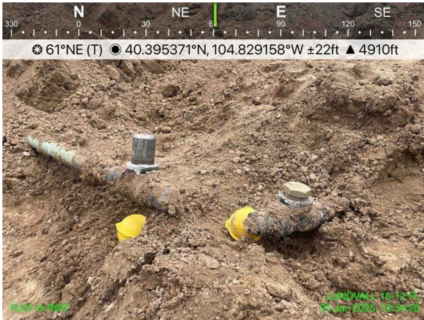
Photo 2: View of flowline separator riser, facing northeast
