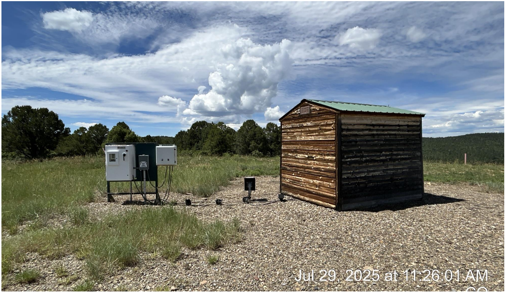
PHOTO 3: WELLHEAD AND EQUIPMENT
