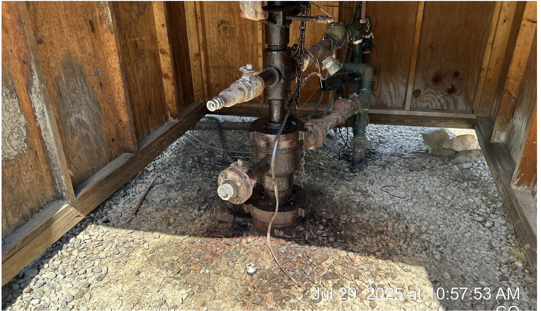
PHOTO 2: IMPACTED SOIL AT WELLHEAD
