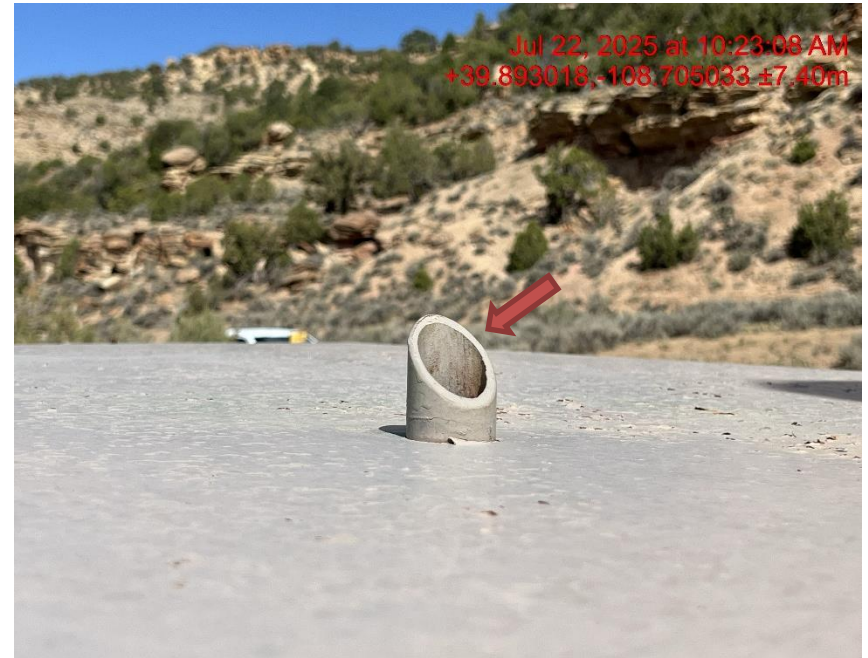
Photo # 0489 PRV vent line does not comply with CECMC pressure safety device rules
