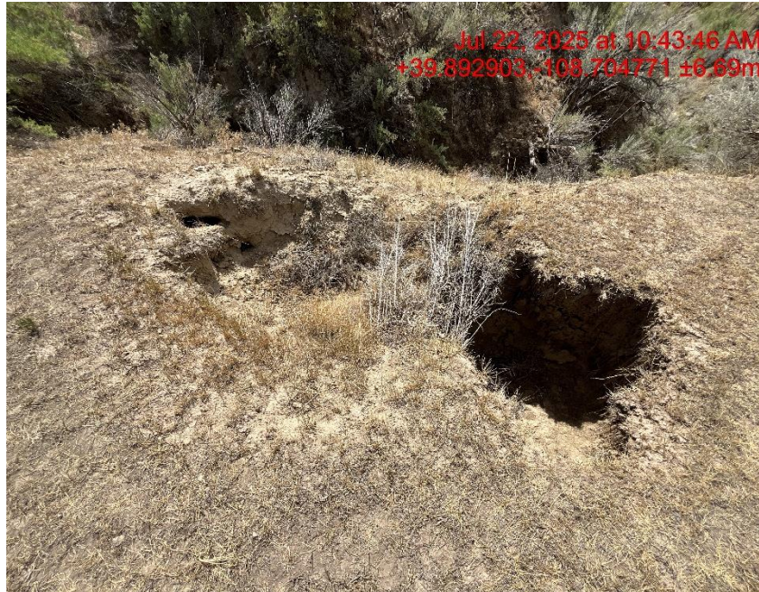
Photo # 0508 Subsidence on south side of location, additionally is a wildlife hazard/personnel safety hazard
