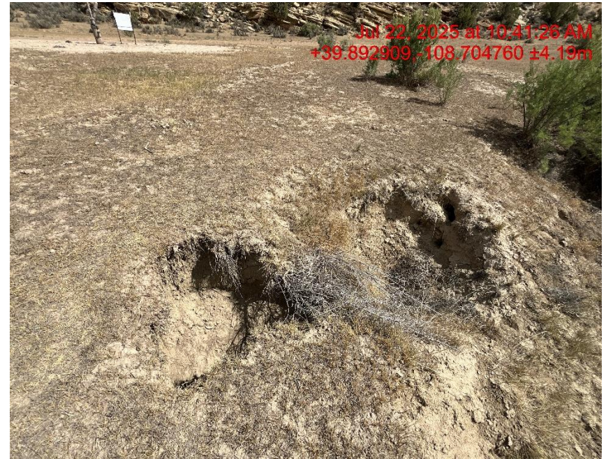
Photo # 0506 Subsidence on south side of location, additionally is a wildlife hazard/personnel safety hazard
