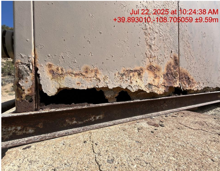
Photo # 0490 Separator housing is damaged and open to wildlife/available for entry by wildlife
