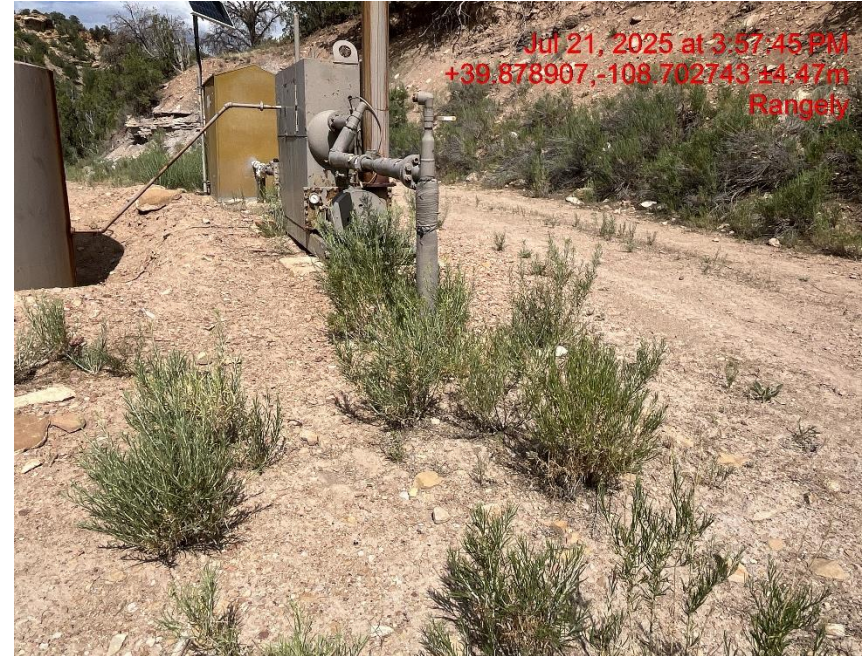
Photo # 0432 Weeds/undesirable plant species surrounding production equipment constitutes a fire hazard
