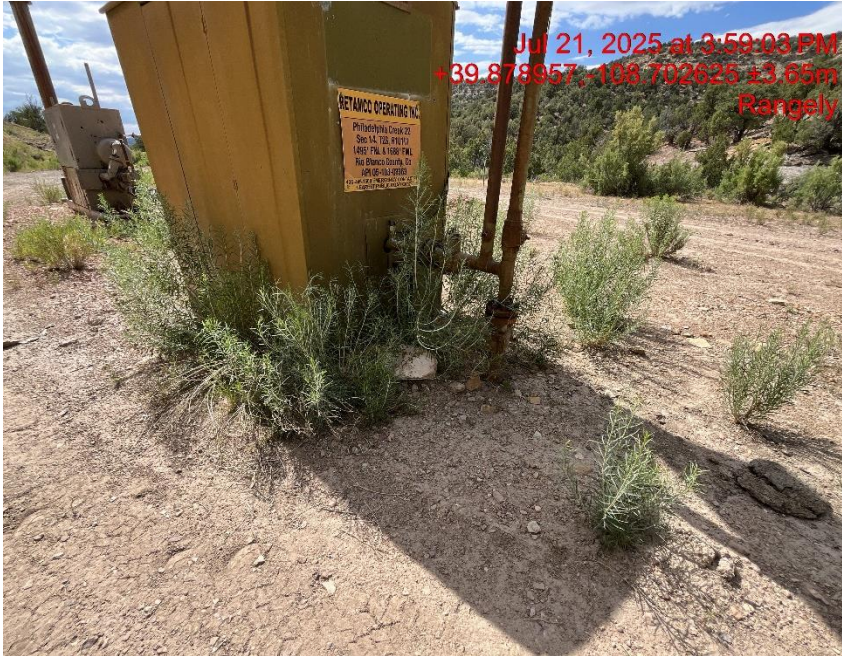
Photo # 0435 Weeds/undesirable plant species surrounding production equipment constitutes a fire hazard
