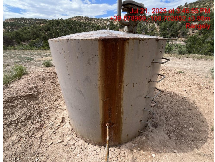
Photo # 0422 Tank showing signs of rust. All in-service Tanks and process vessels will be inspected and maintained
