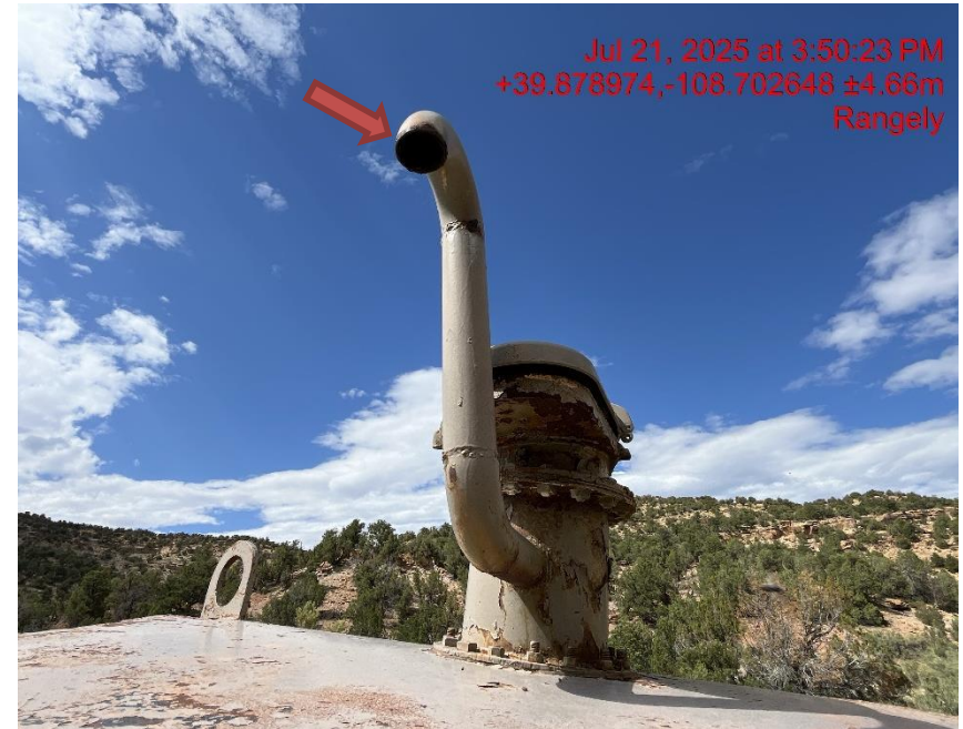
Photo # 0426 Open ended piping/wildlife hazard/available for entry by wildlife
