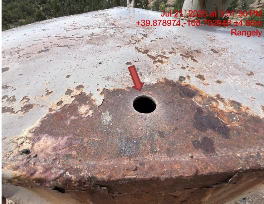
Photo # 0428 Hole in tank/wildlife hazard/available for entry by wildlife
