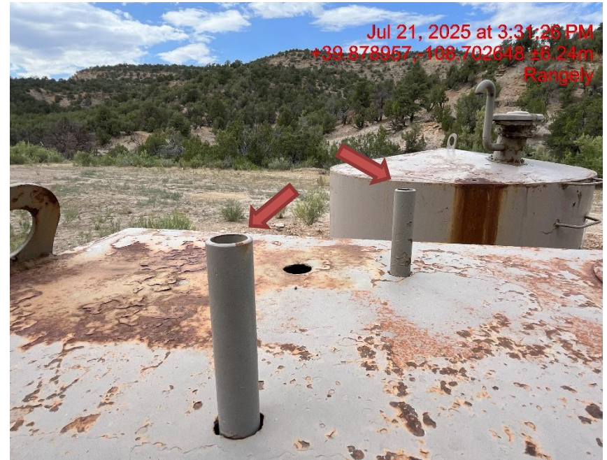
Photo # 0410 PRV vent lines do not comply with CECMC pressure safety device rules
