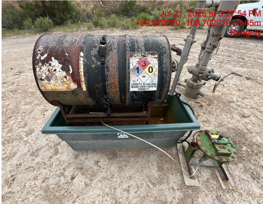
Photo # 0401 Unused equipment - Chemical tank is not in use/unused equipment
