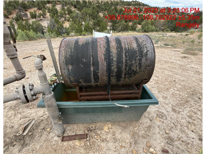
Photo # 0402 Unused equipment - Chemical tank is not in use/unused equipment
