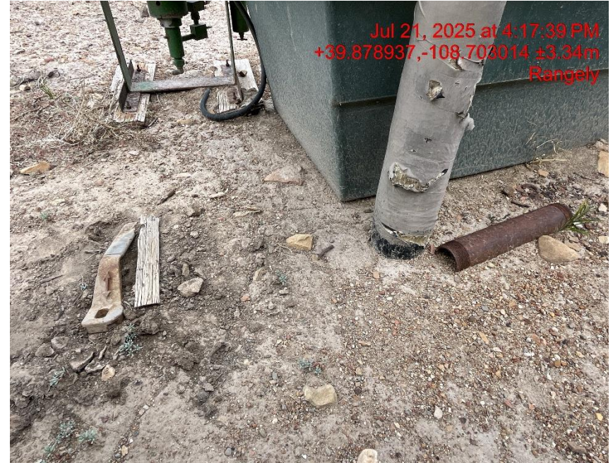
Photo # 0451 Debris on location
