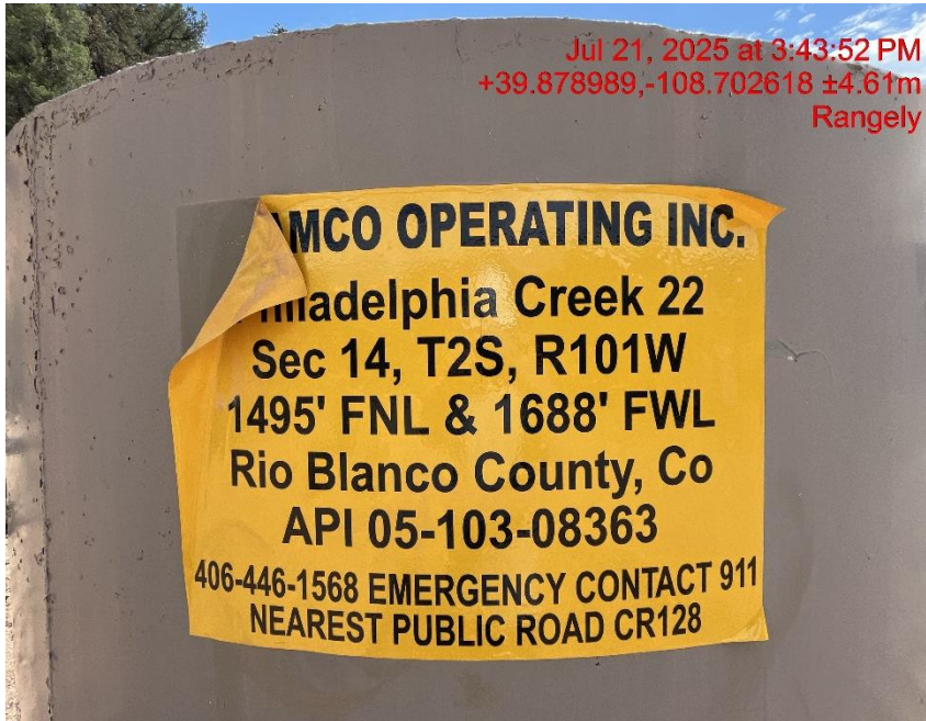
Photo # 0419 Battery sign is in disrepair and lacks quarter/quarter section information/not in compliance with CECMC rules
