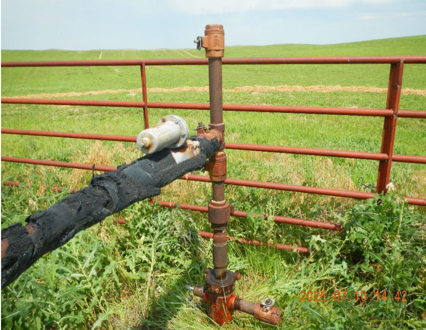
3. View of wellhead tree.
