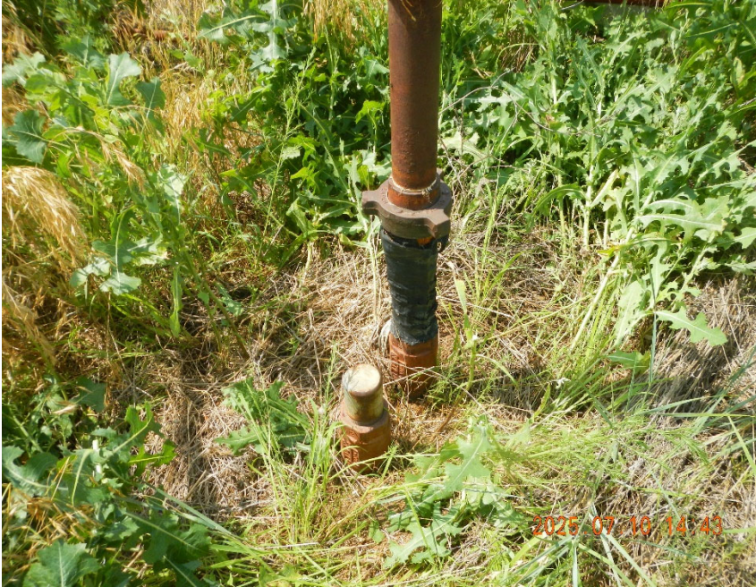
5. View of Flowline Riser with valve and plug wellhead.
