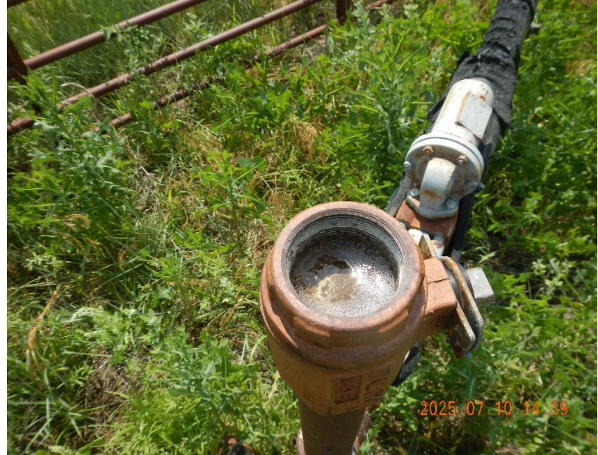
4. View of leaking valve at top of wellhead tree.
