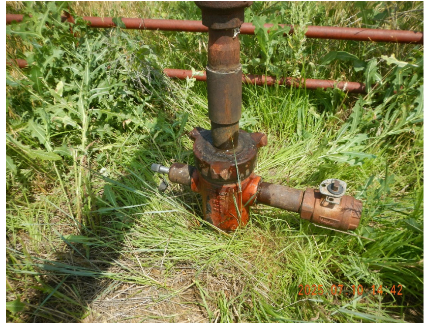
2. View of wellhead.
