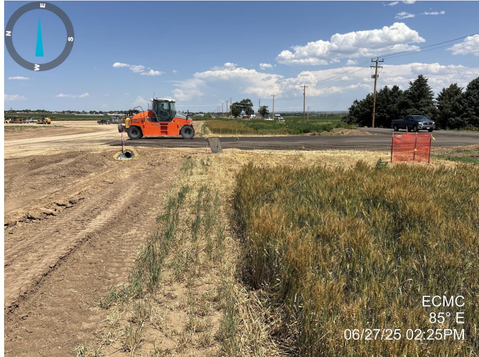
Photo 6. Photo taken of the eastern entrance to the location along the southern perimeter. Photo illustrates a culvert has been installed and the operator was in the process of stabilizing the entrance with road base.
