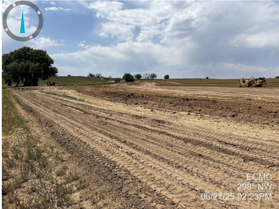
Photo 4. Photo taken from the southern perimeter of the location, facing northwest. Photo illustrates the operator is in the process of stabilizing the working pad surface.
