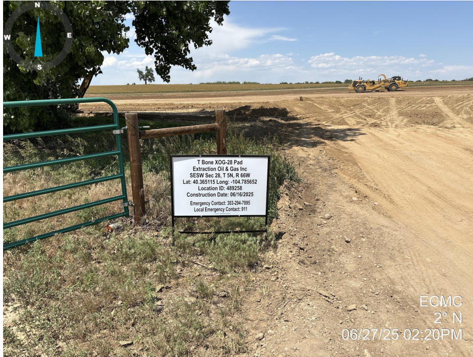
Photo 1. Photo taken from the entrance to the location. Photo illustrates the Operator sign. No mailbox or permits were observed at the time of this inspection.
