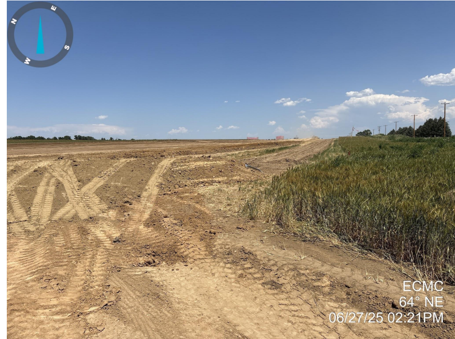
Photo 2. Photo taken of the entrance to the location, facing northeast. Photo illustrates that ditch and berm BMPs have not been installed along the perimeter of the location.
