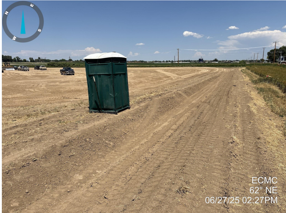
Photo 8. Photo taken from southeastern perimeter of the location, facing northeast. Photo illustrates a porta potty has been stabilized per best management practices. The operator is in the process of installing a ditch and berm along this portion of the location.
