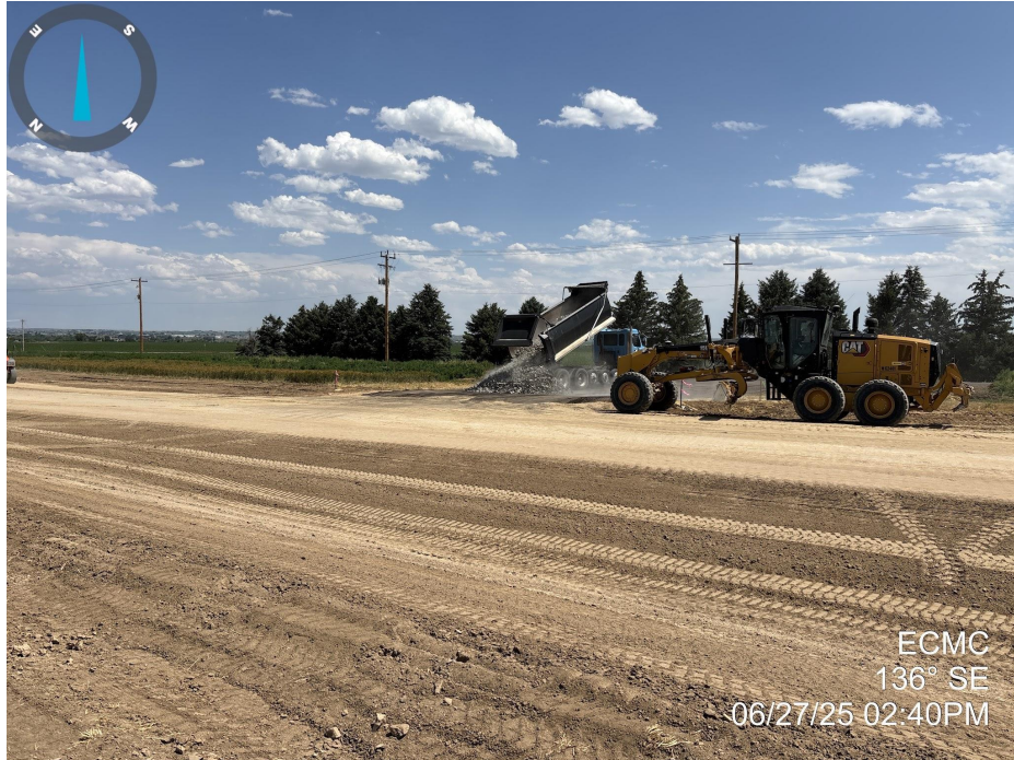
Photo 7. Photo taken of the eastern entrance to the location along the southern perimeter. Photo illustrates that at the time of this inspection rock was being installed to create a vehicle tracking pad.
