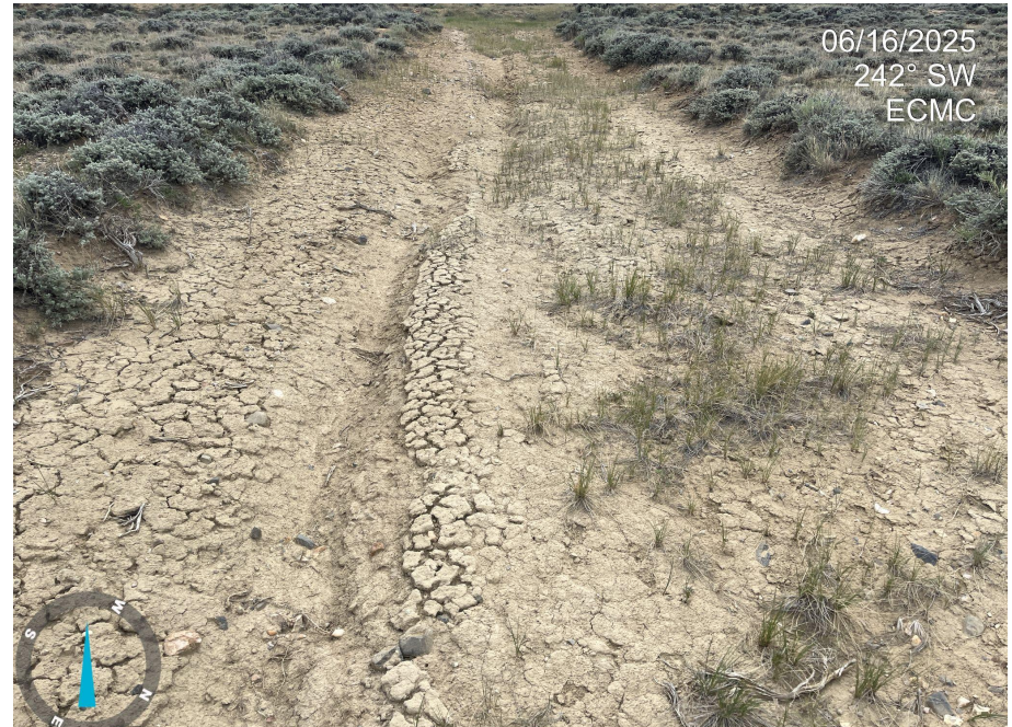
Photo 6. Photos 6-8 taken of the access road, illustrating that the access road is experiencing erosion, primarily in the portion closest to the pad entrance.
