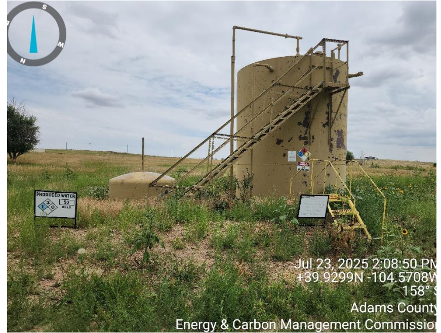
Photo 4 tank battery and equipment
