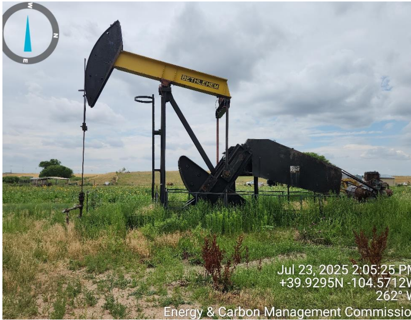
Photo 1 well head and equipment
