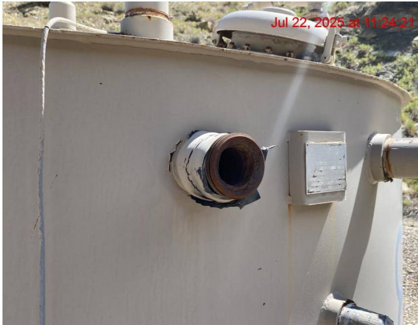
Open-Ended Line on Tank/Wildlife Entry Hazard – Photo #09833
