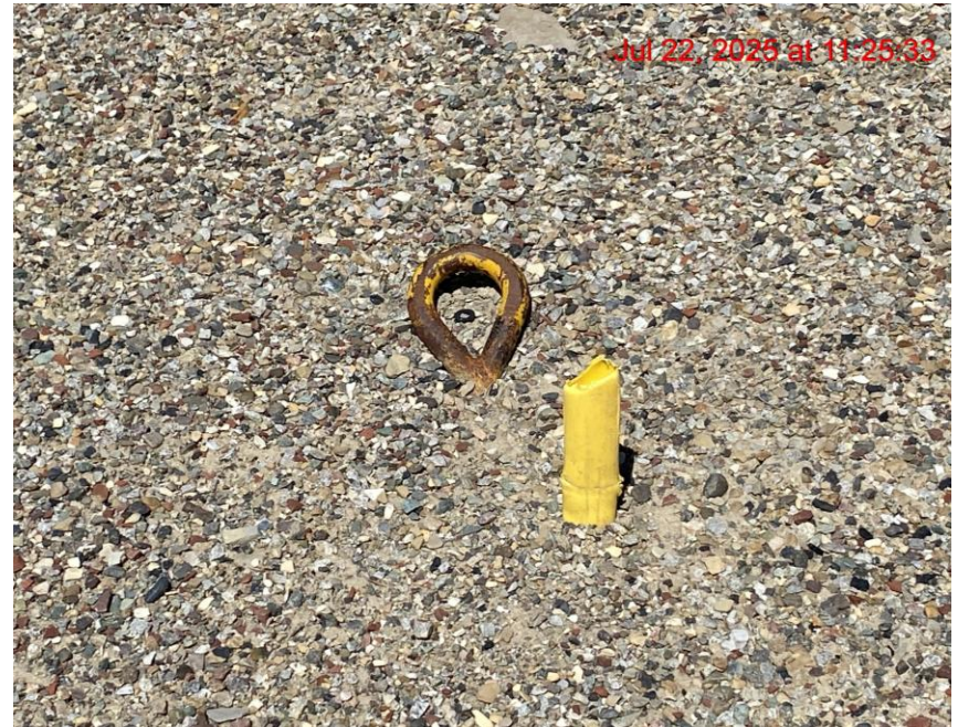
Improperly Marked Deadman – Photo #09836
