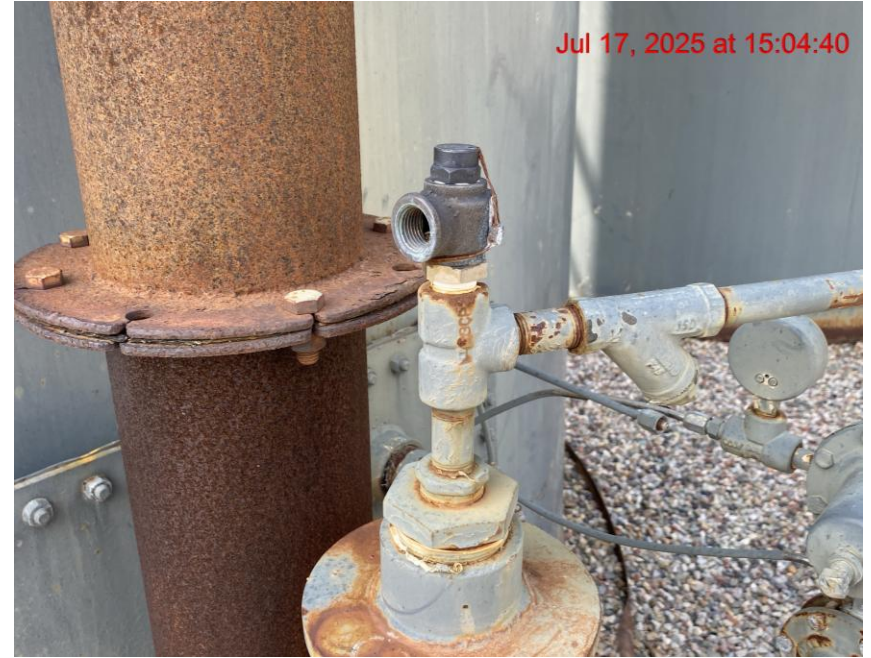
PRV Terminates in Unsafe Manner – Photo #09823
