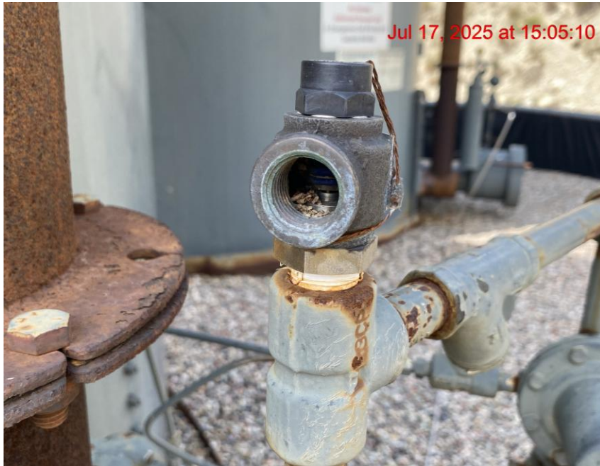
PRV Terminates in Unsafe Manner – Photo #09824
