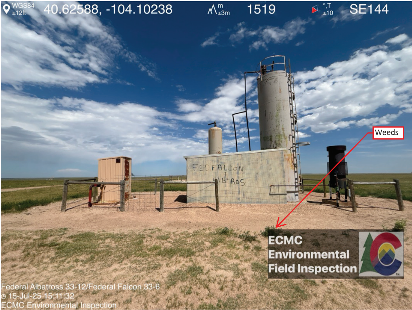
Federal Falcon #33-06 tank battery (Location ID 467686) Meter shed, vertical heater treater, ECD - Fencing adequate Weeds
